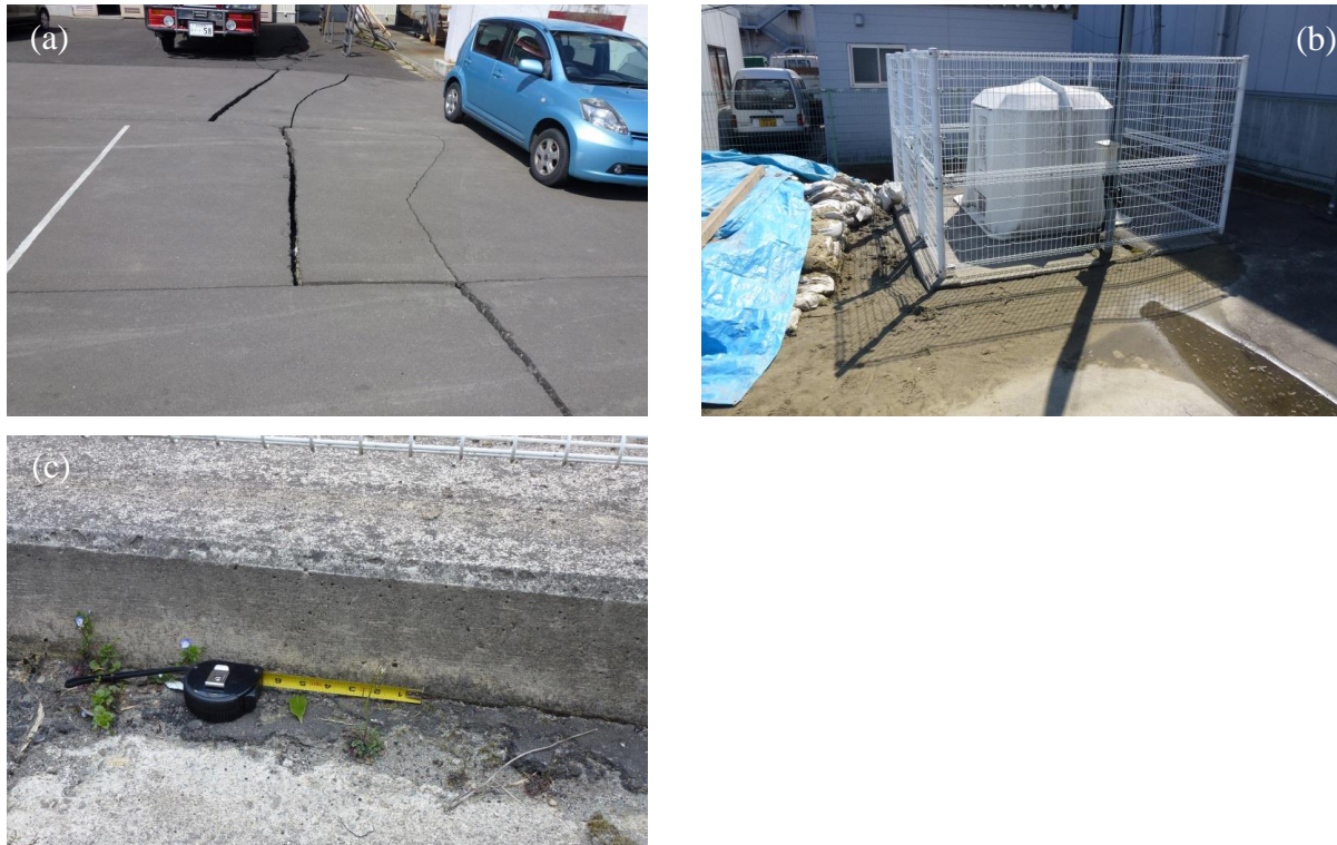
Figure 7.56: Photos showing surficial evidence of liquefaction at MYG013. (a) Cracking in nearby parking lot. Ejecta was swept away before photo. (b) Ejecta surrounding MYG013 instrument (c) Possible evidence of instrument pad settlement. Images courtesy of Steve Kramer, GEER, taken on April 12, 2011.
