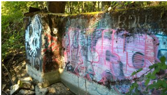
Figure 57 Graffiti art on concrete foundation
