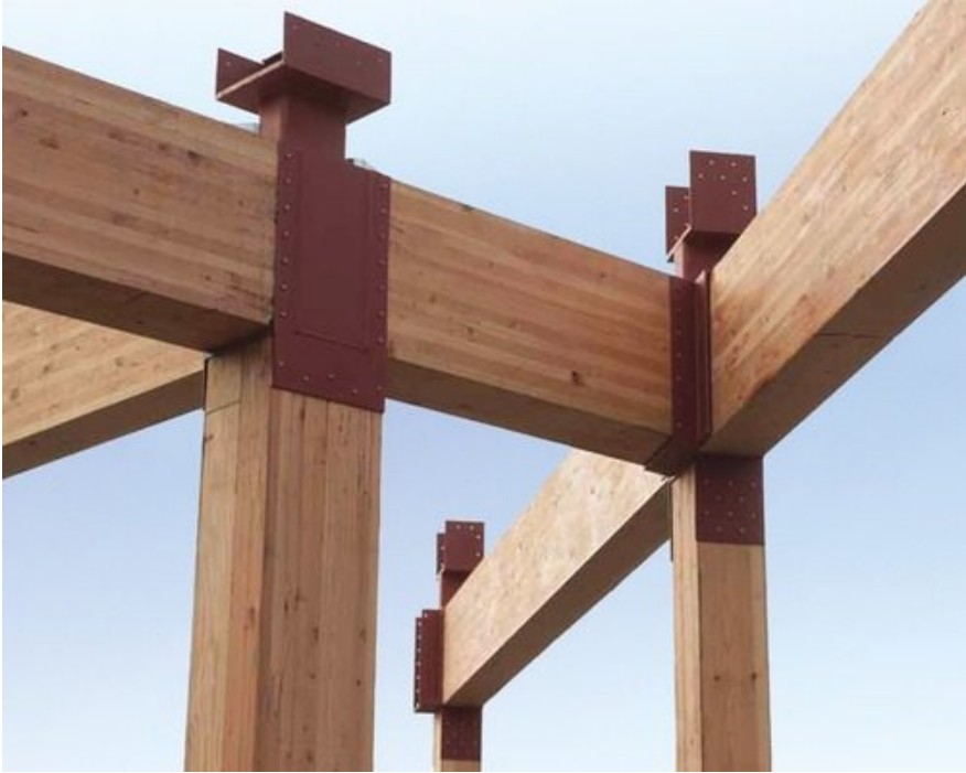
Figure 2.1: Steel connectors are located at each connection point.(Bullitt Center, Seattle, WA, USA; 2011)
