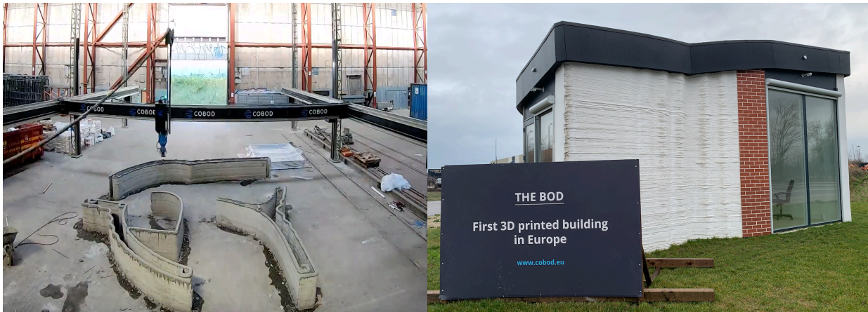
Figure 4.11: A clip from a time-lapse by COBOD of their test “BOD” structure (cobod.com/videos). Figure 4.12: The completed BOD structure in Nyhavn area of Copenhagen, Denmark (Photo by author).
