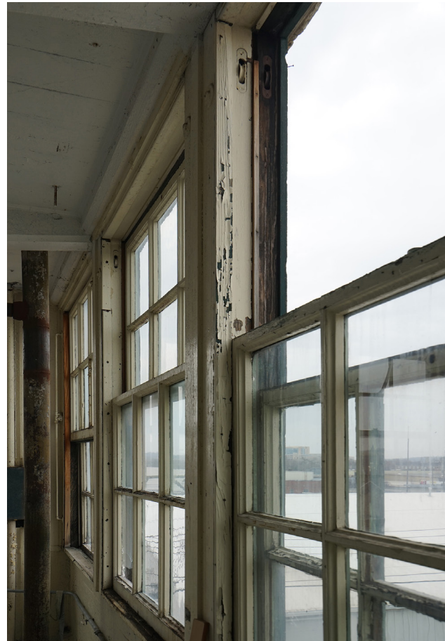
Fig. 4.1 View of windows on the west wall of the southwest corner of the Dayton Motor Car Company building showing window conditions, mullion thickness, and frame thickness. Photo: April 2015, by author.
