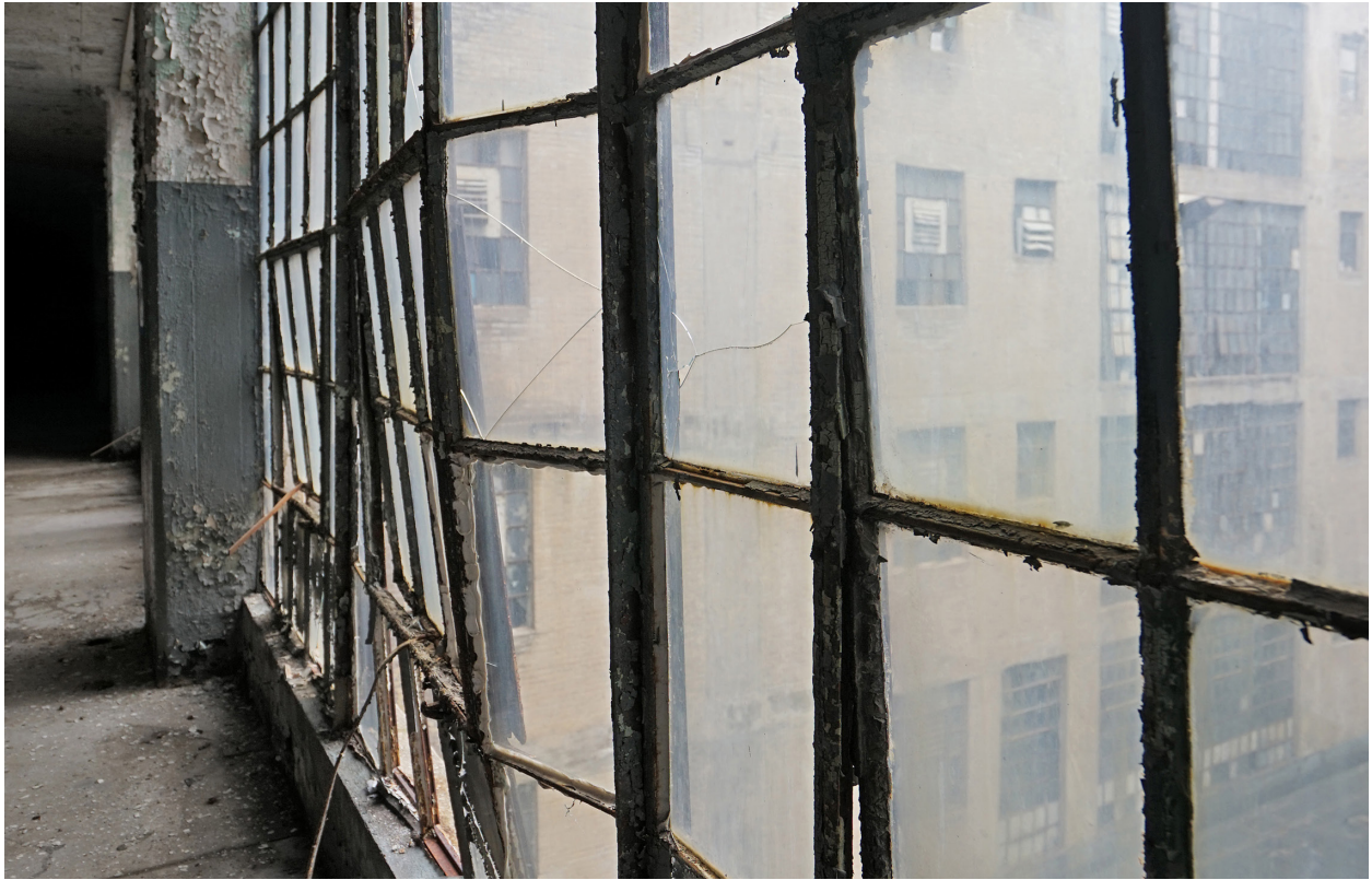
Fig. 3.49 Detail of windows showing damage, April 2015. In addition to rust and surface deterioration, many windows frames are failing. Photo by author.
