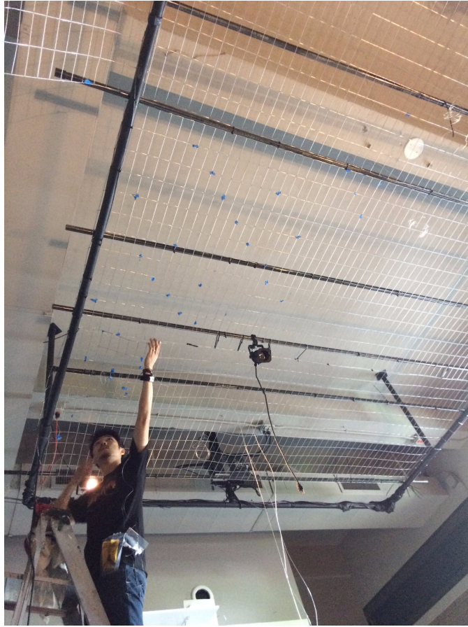
Figure 7.42: Setting up the ceiling wire mesh at Jack Straw New Media Center
