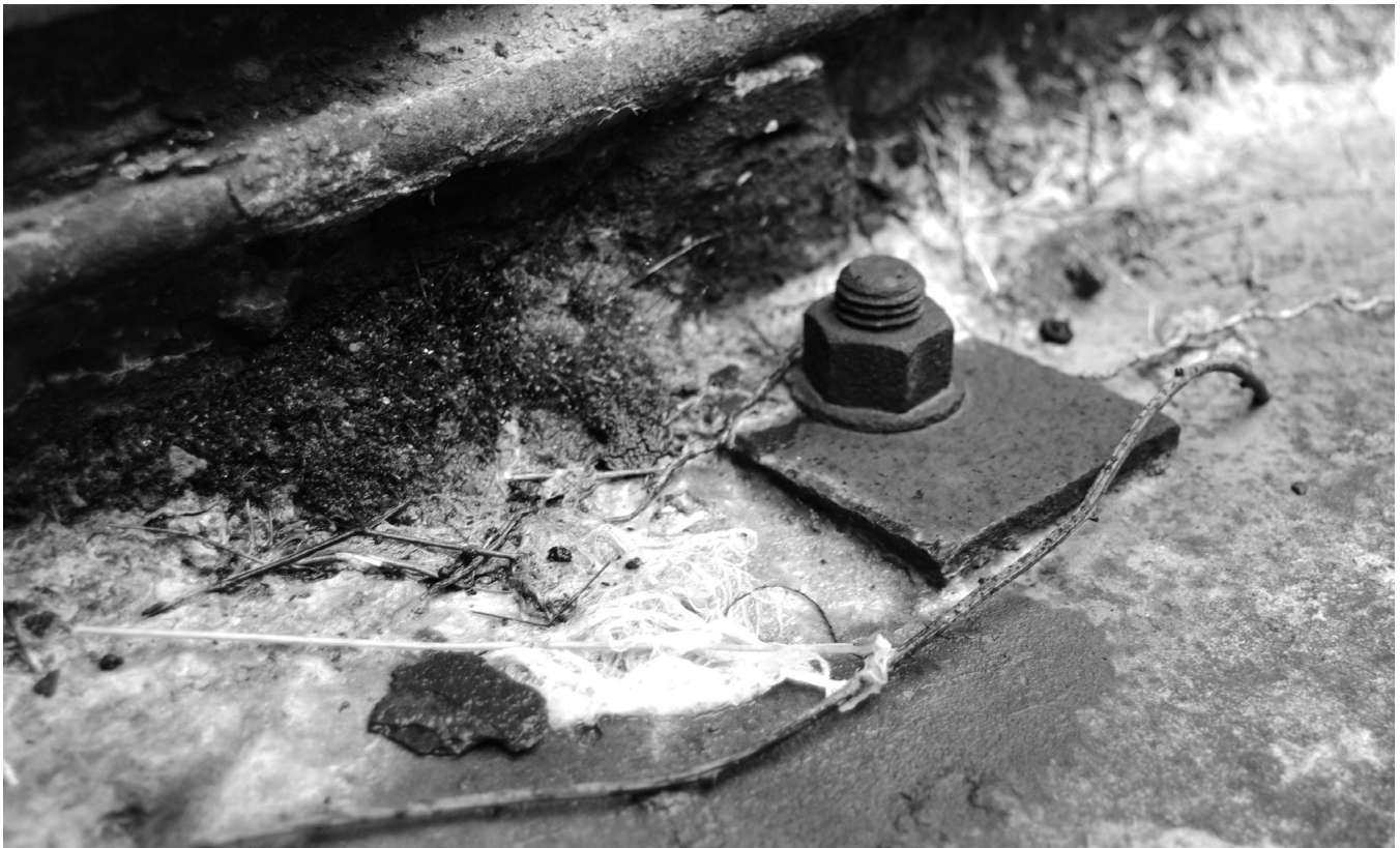
9. residue on coal silo, fitchburg
