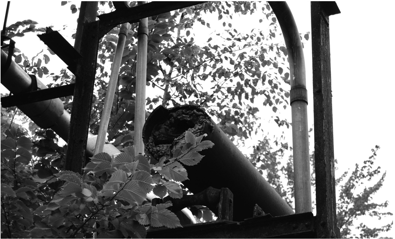
10. disconnected steam pipe, central steam plant in fitchburg
