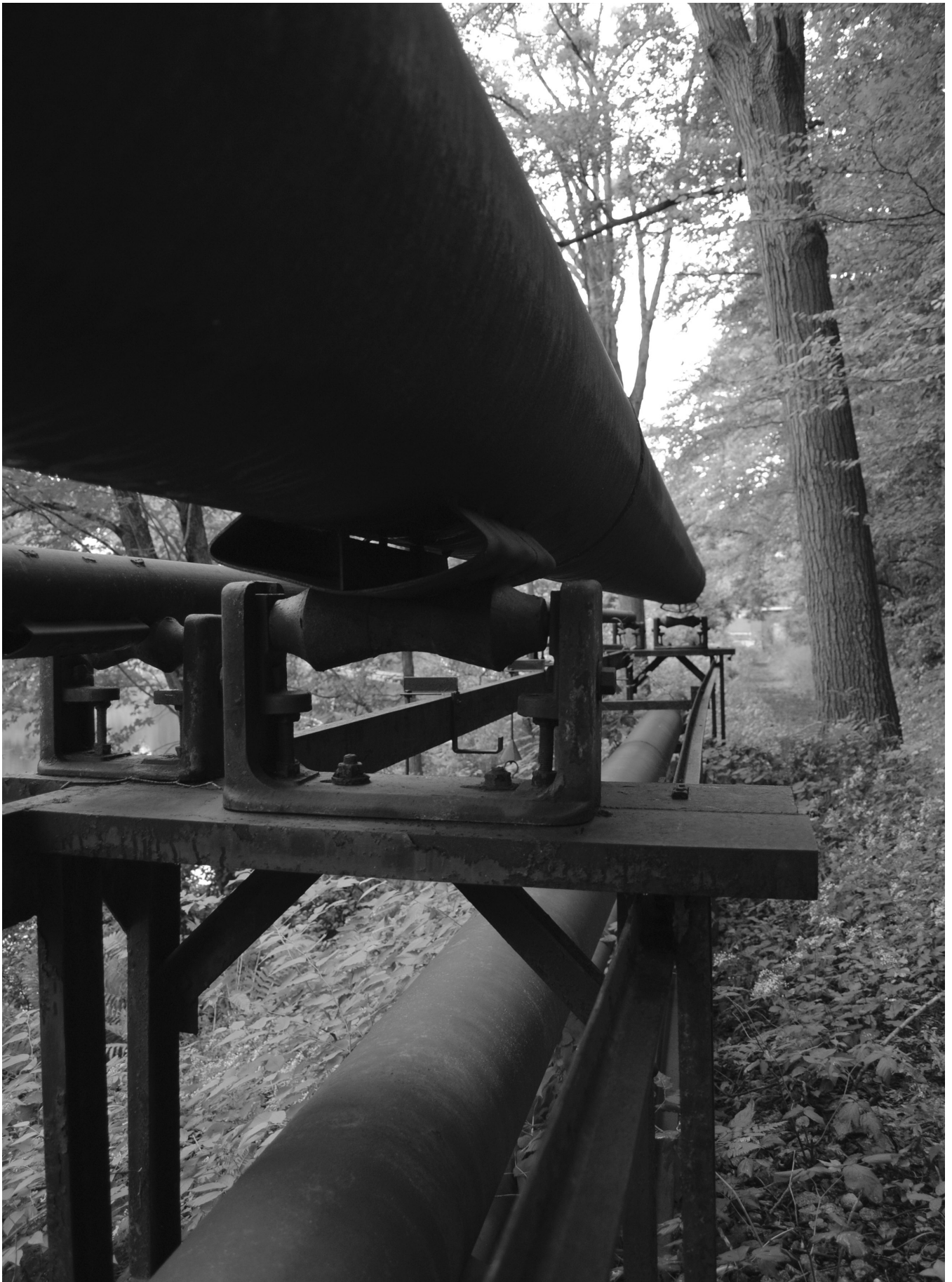
11. steam lines in fitchburg
