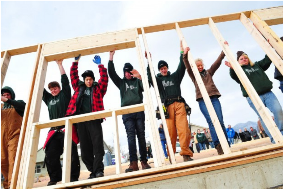
Figure 17: YouthCare's YouthBuild program employs the help of troubled homeless teens to build affordable housing units in their local community.
