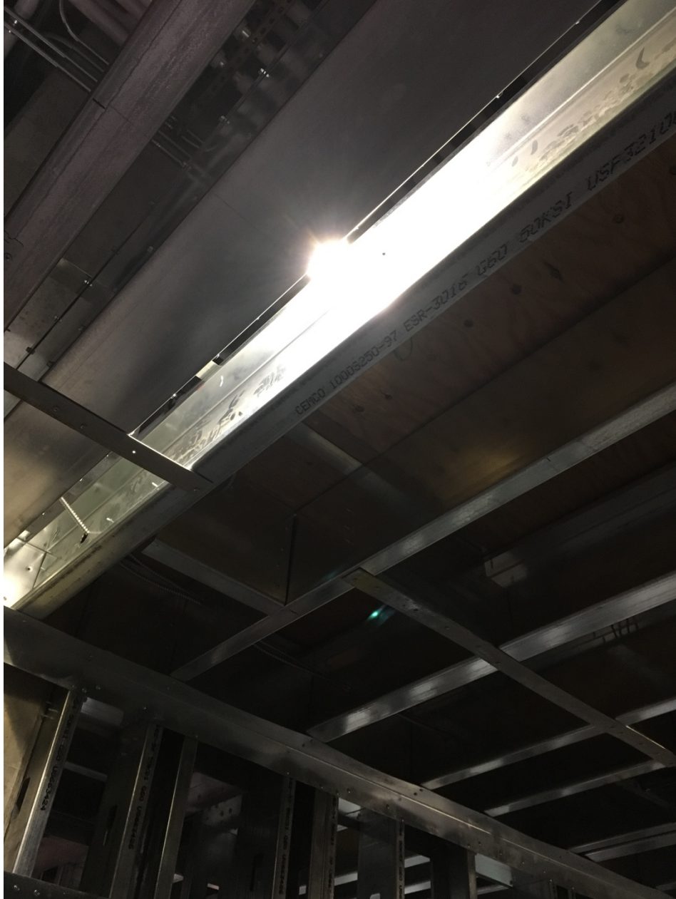
Figure 32: Corridor D: FM2 Blocked by Steel Framing
