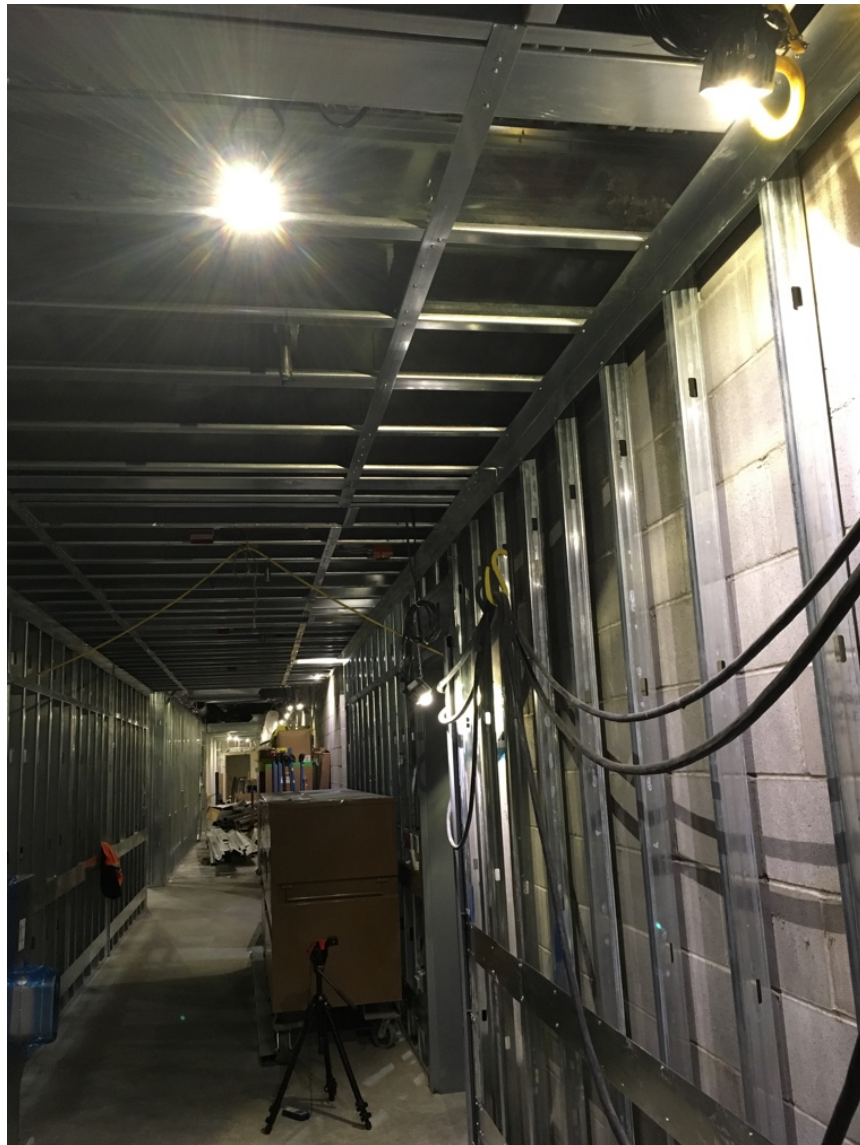
Figure 30: Lights High Above Framing and Shadows Cast by Tool Box
