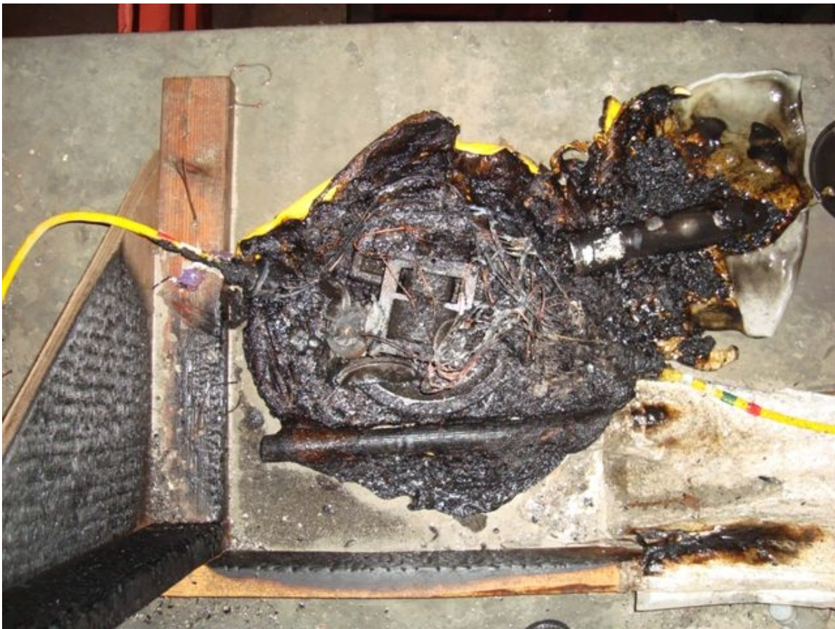
Figure 8: Bravern Wobble Light Fire (Source: Skanska)
