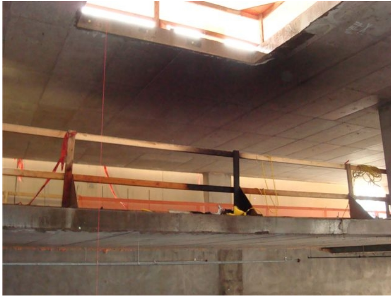
Figure 9: Bravern Wobble Light Fire (Source: Skanska)
