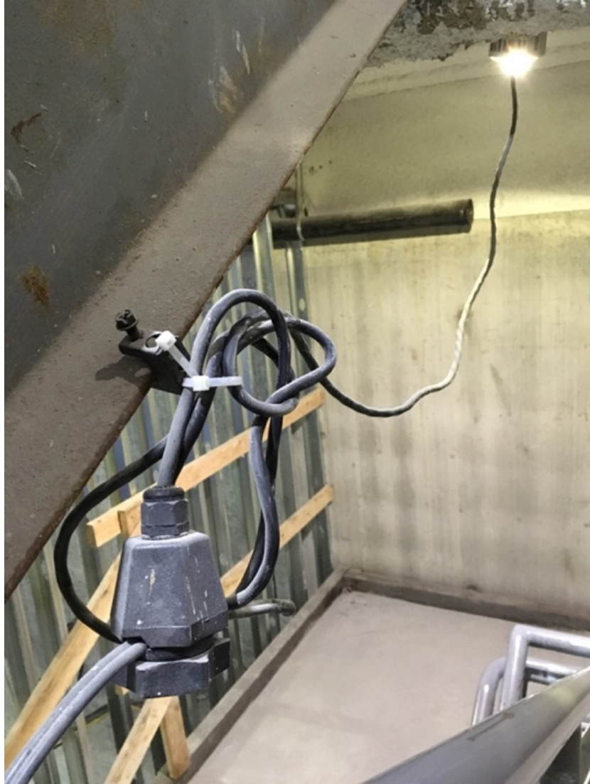
Figure 17: FM2 and Twist-Lock Connector at ARCF Stairwell
