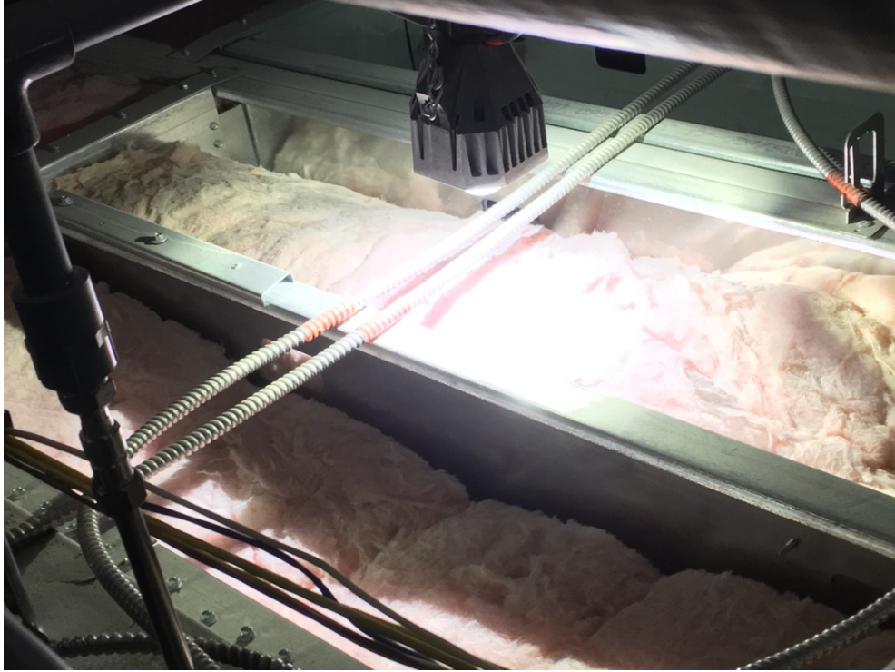
Figure 33: FM2 in Interstitial B02 Blocked by Insulation
