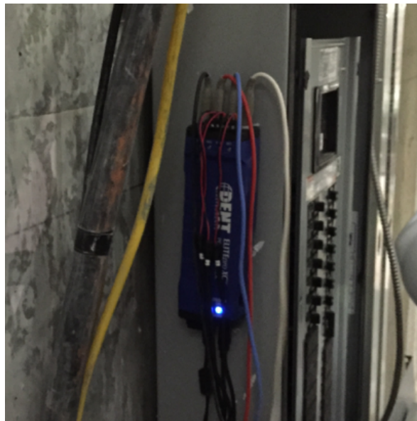
Figure 20: Installed Energy Logger at ARCF (Source: Smith. 2016)
