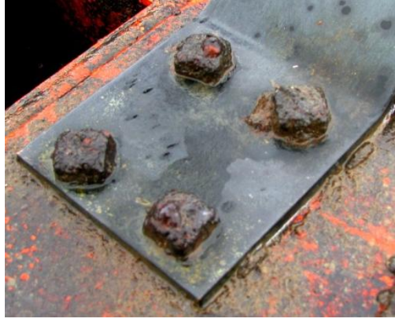
Figure 25: Galvanic corrosion due to coupling of steel bolt to the bronze spring.
