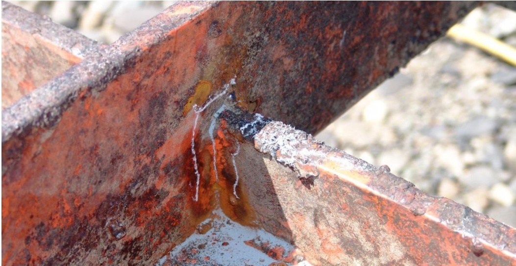
Figure 8: The first round of magnetic particle testing was performed through the paint. The grey powder serves as a strong indication that there is a crack in the weld. This proved to be true after grinding into the weld.
