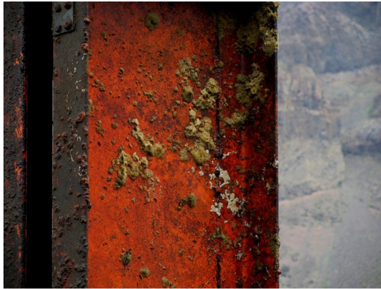
Figure 24: Example of biological growth.
