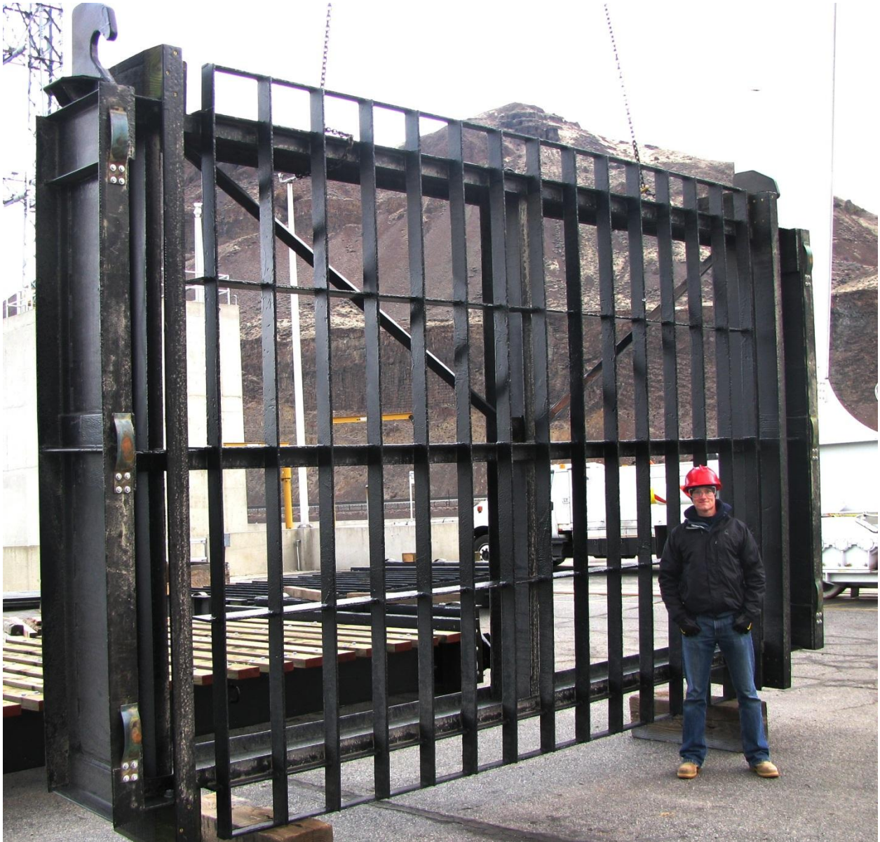
Figure 41: Rehabilitated trashrack. The new diagonal braces were installed and the structure was sandblasted and painted black. Tim Scheumann is standing in front of the trashrack.
