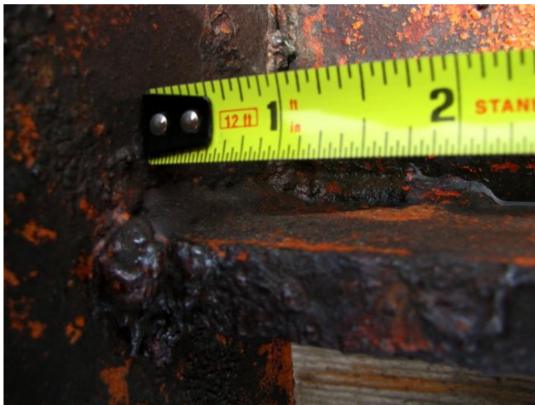
Figure 20: Corrosion deposits along a welded joint.
