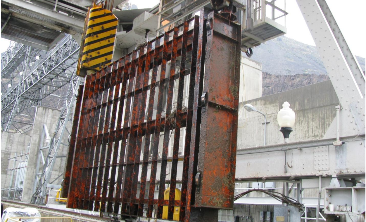
Figure 4: Steel framed trashrack with vertical steel rackbars.
