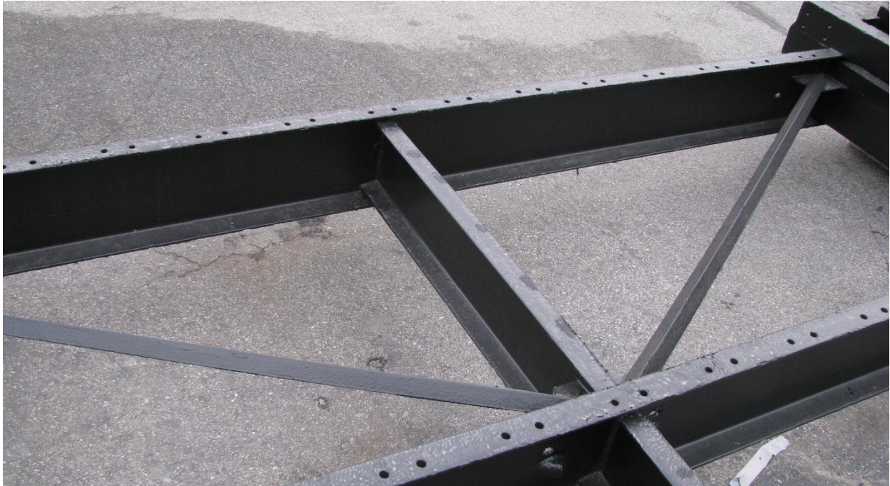
Figure 40: Rehabilitated trashrack demonstrating the new diagonal braces. The angle iron braces were installed with the elbow of the angle pointing directly into the flow.
