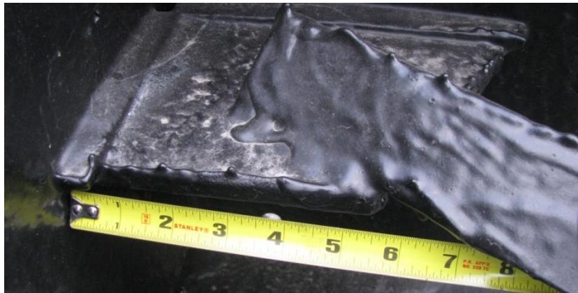
Figure 12: The protective layer of paint was applied unevenly and dripped in many locations. This was likely do to a rushed application process which resulted in uneven layers and was accentuated by the fact that it was applied at an improper ambient temperature.
