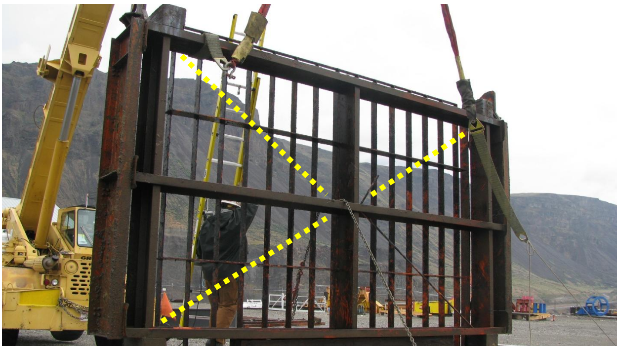
Figure 6: Each trashrack should have four diagonal tie rods to provide stability when moving the 7,000 pound structures. This picture is an example of one rack which is missing three of the tie rods (locations identified in yellow) and the one remaining rod was very loose.
