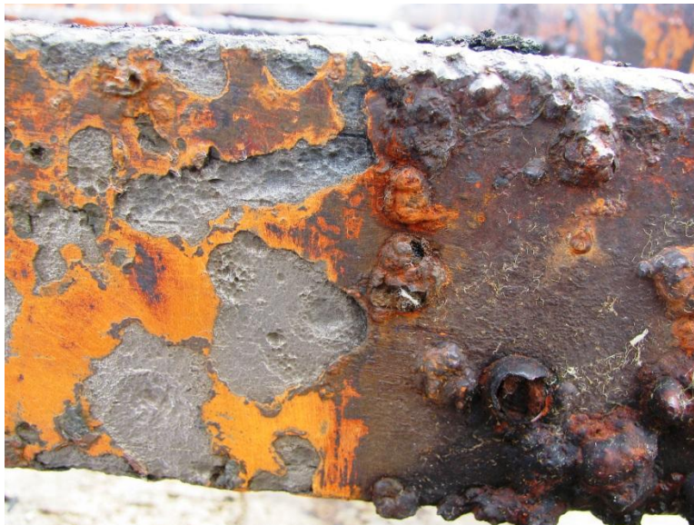
Figure 7: This picture shows a common instance of tubercles as found on the trashracks (right) and the pits which had formed under the tubercles (left).
