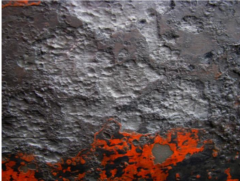
Figure 19: Corrosion damage under a surface covered with tubercles.
