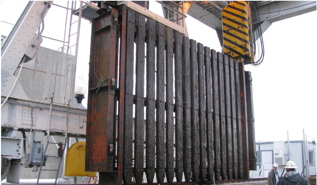
Figure 5: Steel framed trashrack with vertical wood rackbars.
