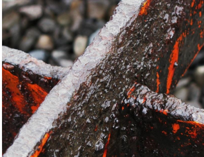
Figure 22: Erosion corrosion damage of leading edge.
