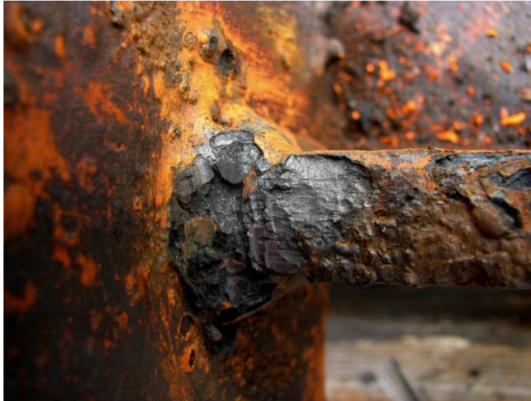
Figure 21: Corrosion damage after the tubercles have been removed from the weld.
