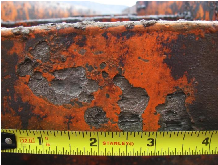
Figure 18: Corrosion damage under a few individual tubercles.
