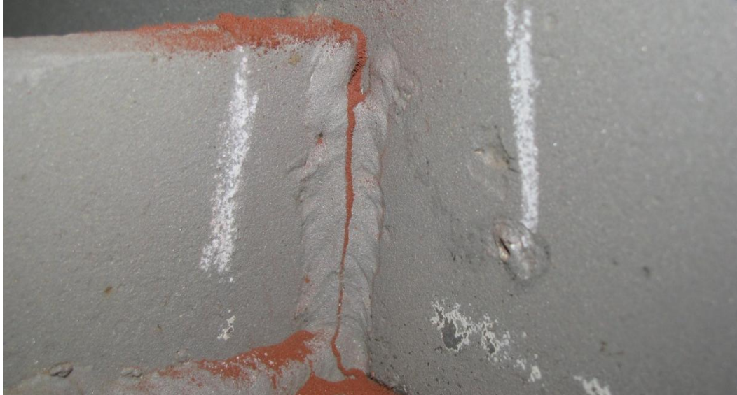
Figure 10: Magnetic particle testing was performed a second time after the trashracks were sandblasted. Red powder was used here to identify the crack.
