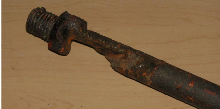
Figure 26: Fretting corrosion evident on the steel tie rod.
