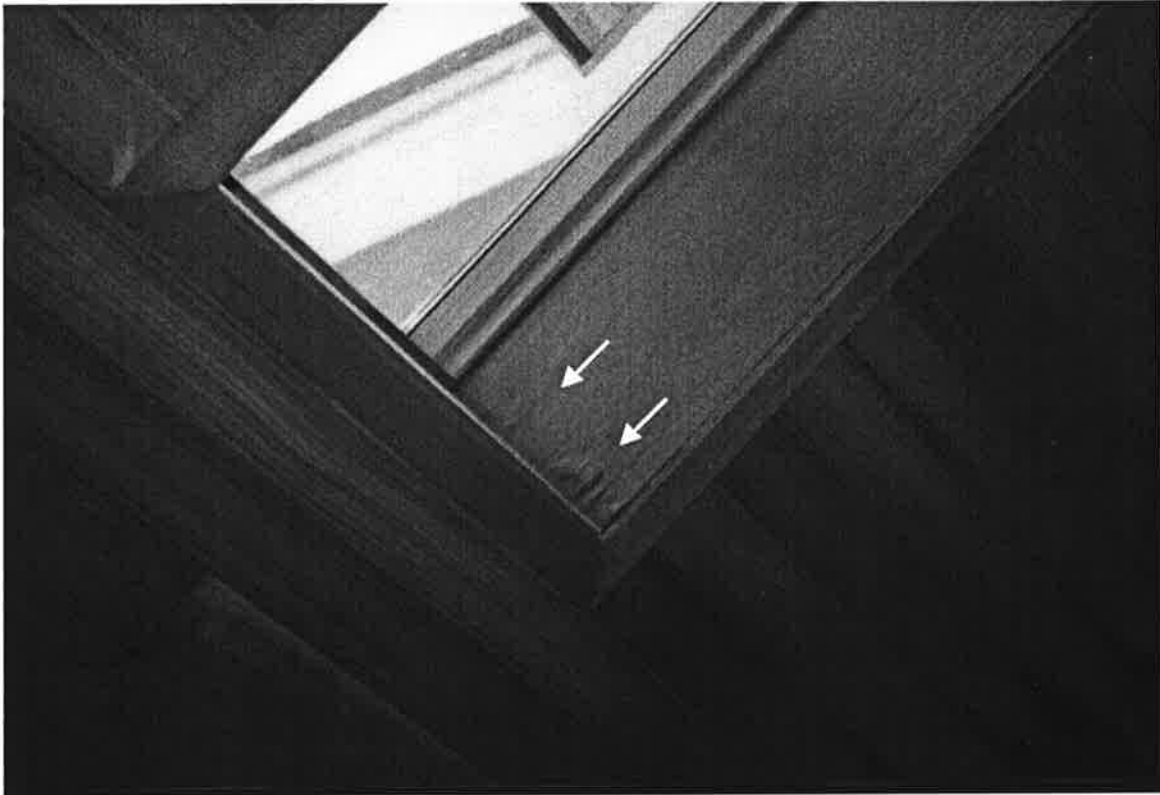
Figure 147. Damage due to poor skylight installation.
