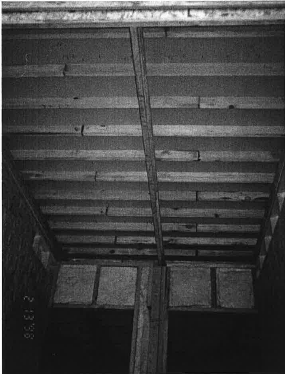
Figure 25. Incorrect I-joist spacing and improper ceiling joists.
