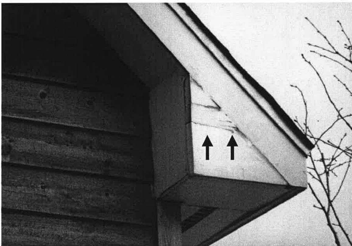
Figure 13. Product quality and paint failure.
