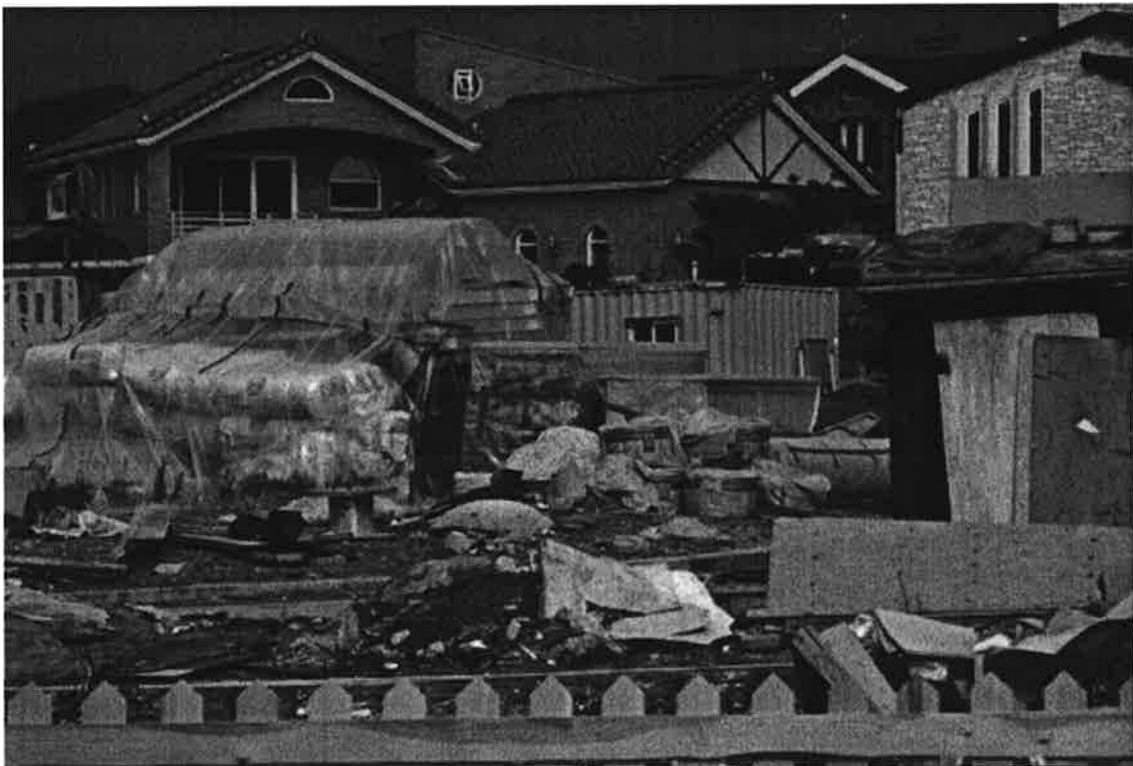
Figure 27. Inadequate site storage of building materials.
