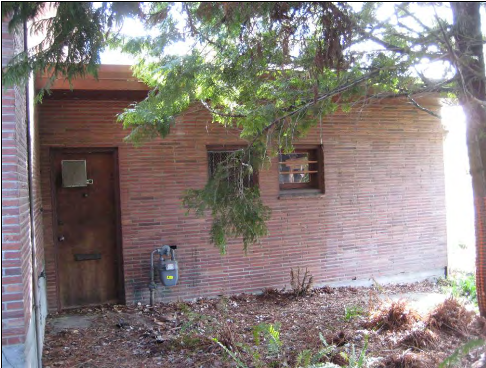
Fig. 19 Above, a detail view of the west façade of accessory building at south end of former apartment building.
