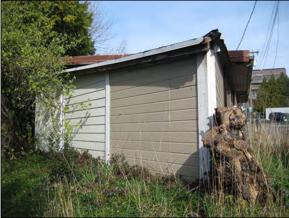
Fig. 21 Above, view north from the southeast corner of the property, showing the accessory building.
