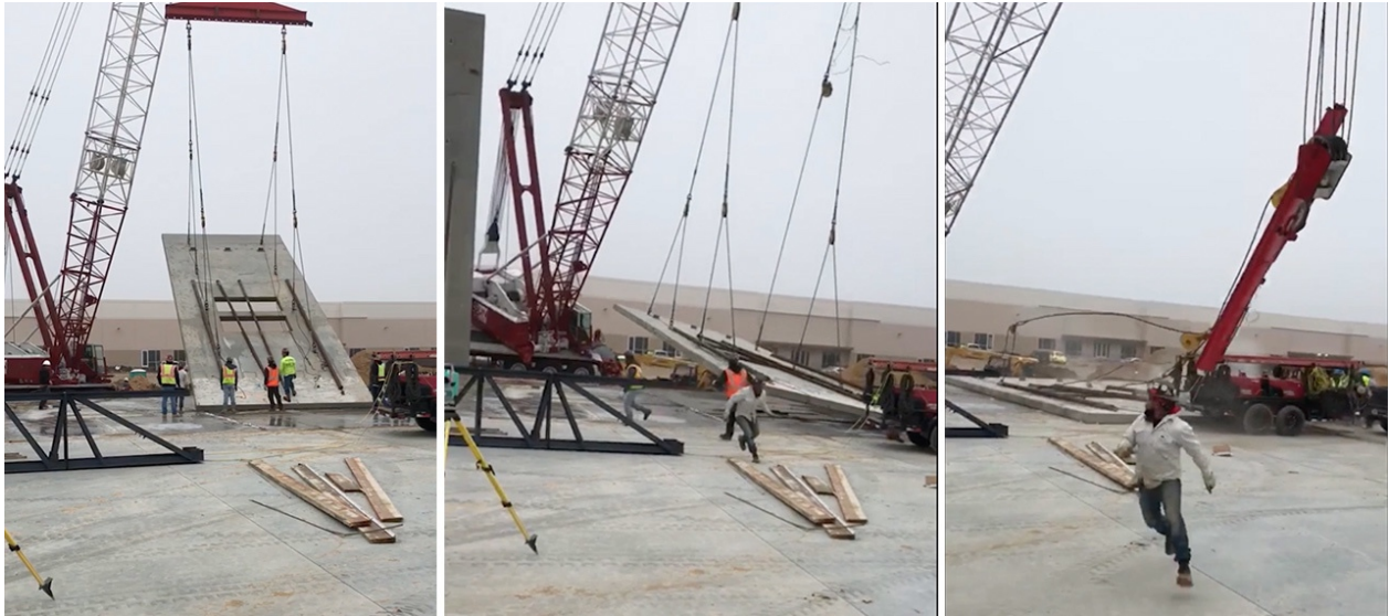
Figure 2. What could go wrong: sequence of a construction accident in Austin TX, involving a precast wall component. Retrieved from: https://youtu.be/Mn6PYOG6sWw .
