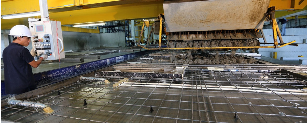
Figure 30. Highly controlled fabrication of precast wall panels. Source: Tekla. Retrieved from: https://www.tekla.com/solutions/precast-fabricators/fabrication .
