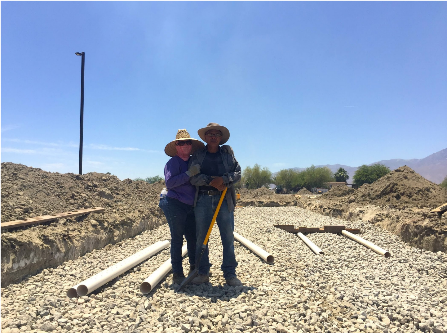
Figure 0.2 Image of Hermelinda Tejas and Ramón Zaragoza building a septic system in their Polanco Park.
