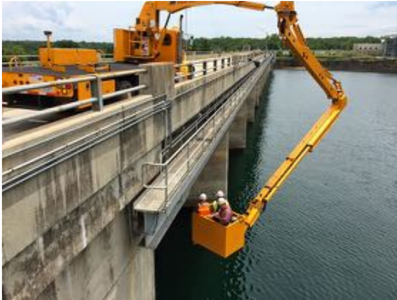
Figure 1.1: Typical damage assessment by the inspection team
