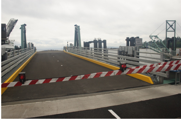
FIGURE 13. THE ENCLOSED HYDRAULIC CYLINDER OF THE H-SPAN, VEHICLE TRANSFER SPAN.
