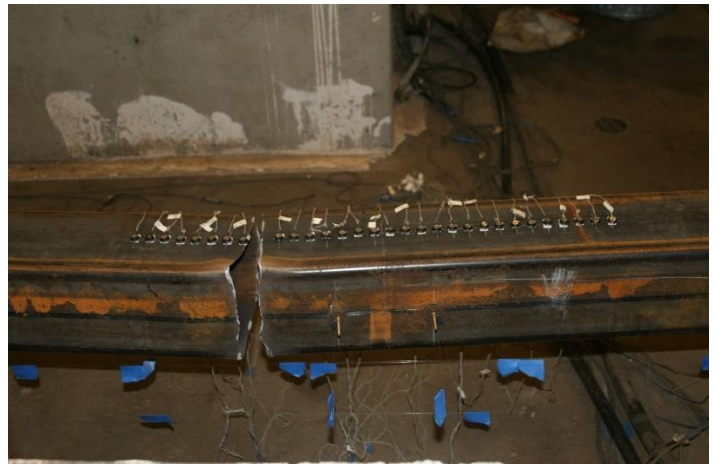
Brace Fracture: 1.62" T1 cycle
