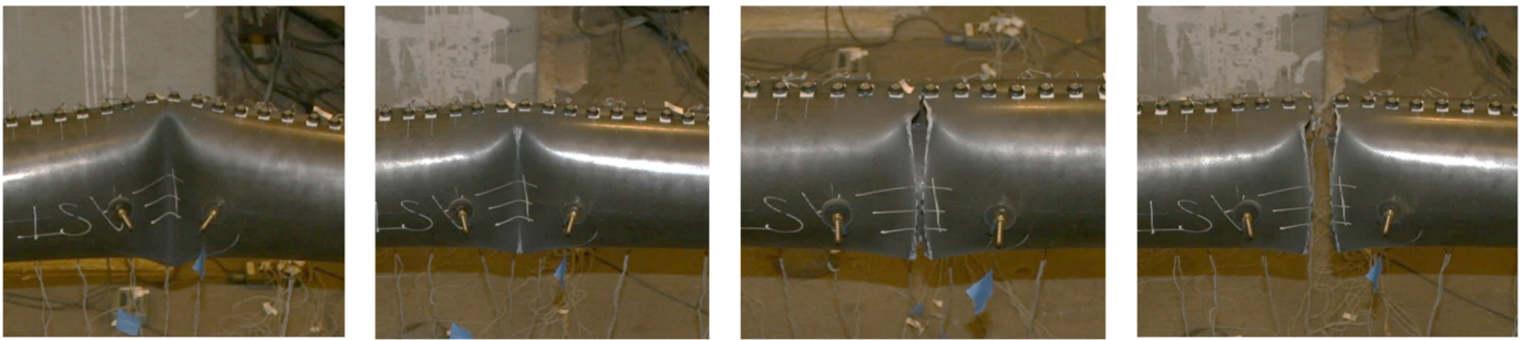
Figure 1.3 Progression of Brace Deformation and Damage at Brace Midspan – Round HSS
