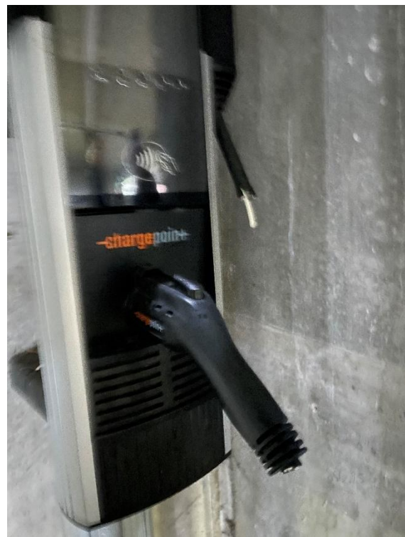
Figure 20: Damaged EV Charging Devices
