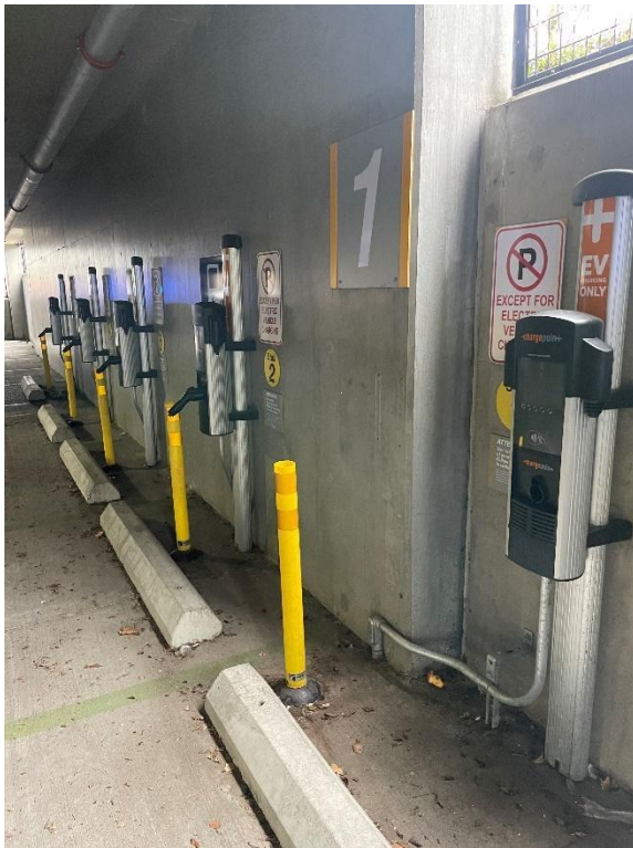
Figure 21: Damaged EV Charging Devices
