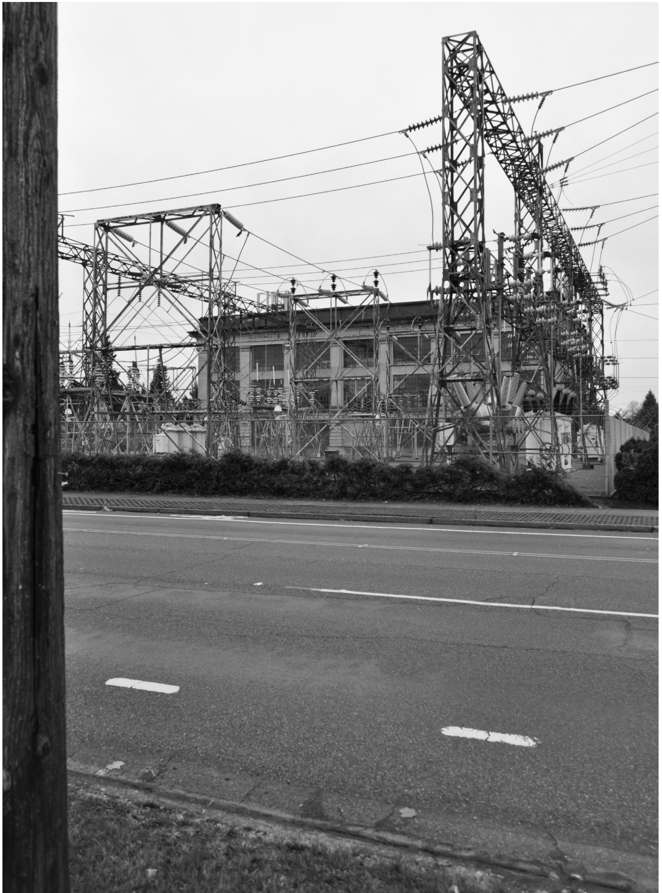
8 figure 1. cushman substation, tacoma wa
