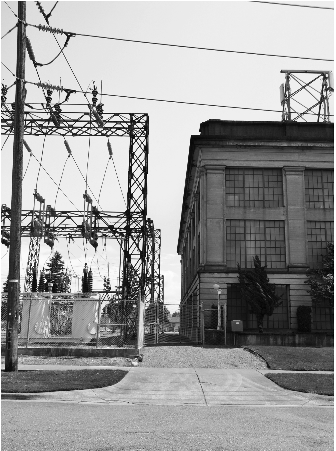
24 figure 13. cushman substation and steel lattice framework
