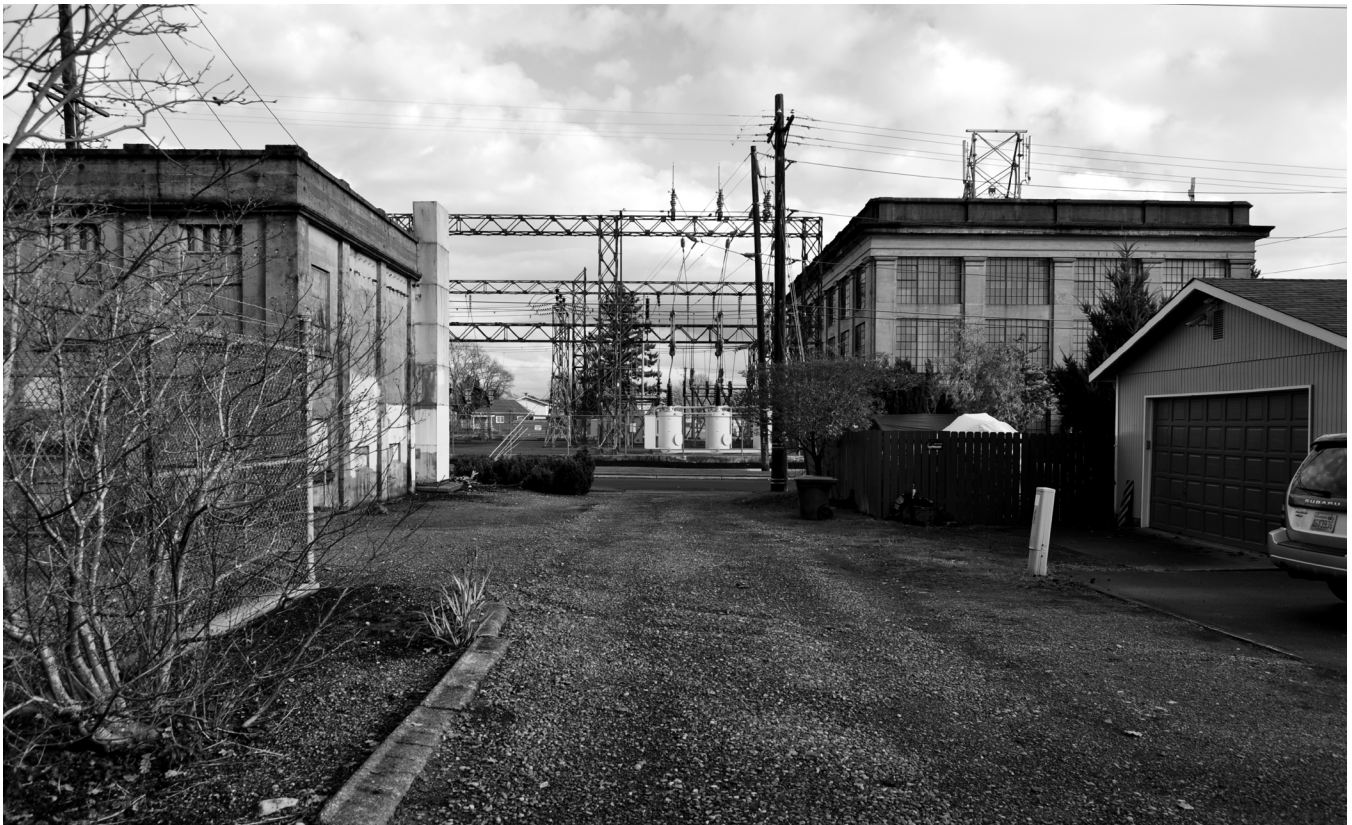
figure 2. cushman substation, adams substation in foreground
