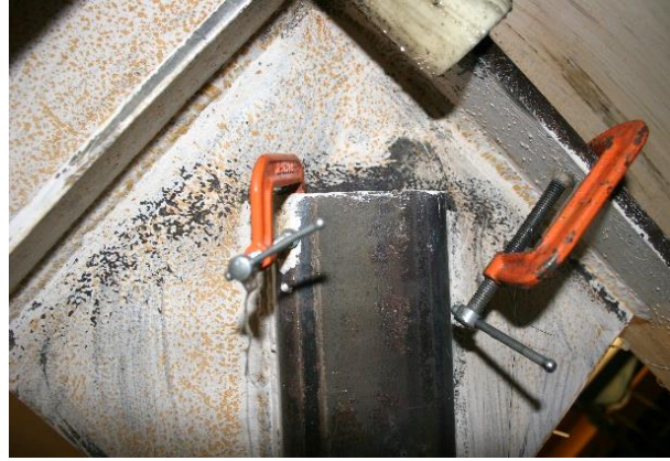
Figure 4.38 Beam Midspan Gusset Elliptical Yielding (SW) 0.83% drift
