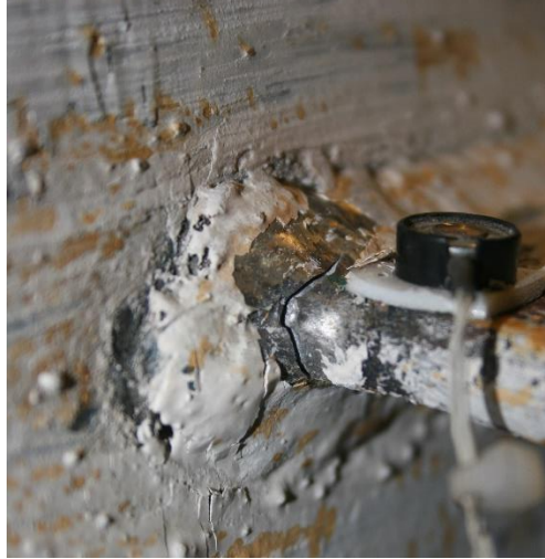
Figure 4.6 Weld crack in gusset plate-to-beam interface weld
