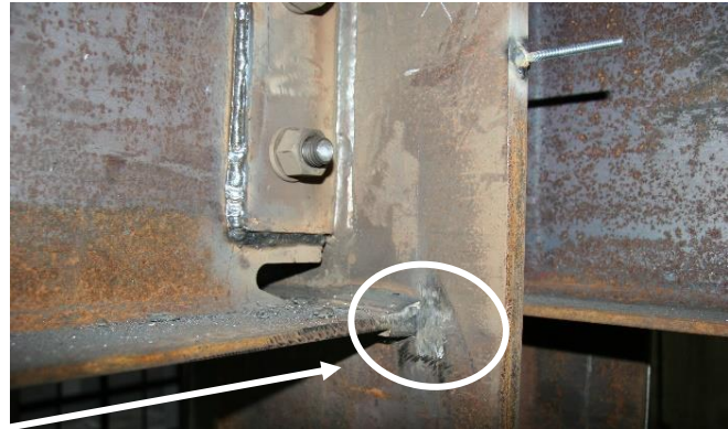
(b) cut and ground weld runoff on bottom flange weld
