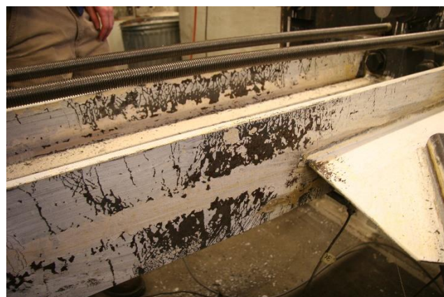
(b) Chevron 2 north column yielding
