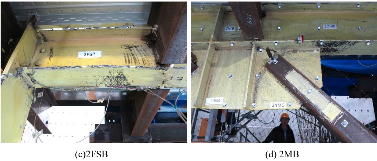
Figure 6.31 2 nd story damage at 1.35% roof drift
