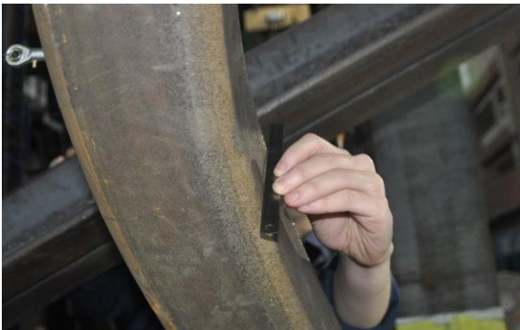
(a) 1NBr at +2.25% roof drift with minimal cupping
