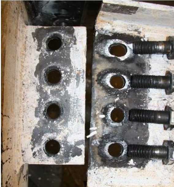
Figure 4.31 S Beam web bolt hole elongation
