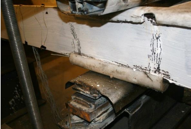
Figure 4.37 Beam Top Flange Yielding at Stiffeners 0.7% Drift
