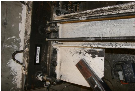
Figure 4.28 N col yielding and buckling @ +3.3%
