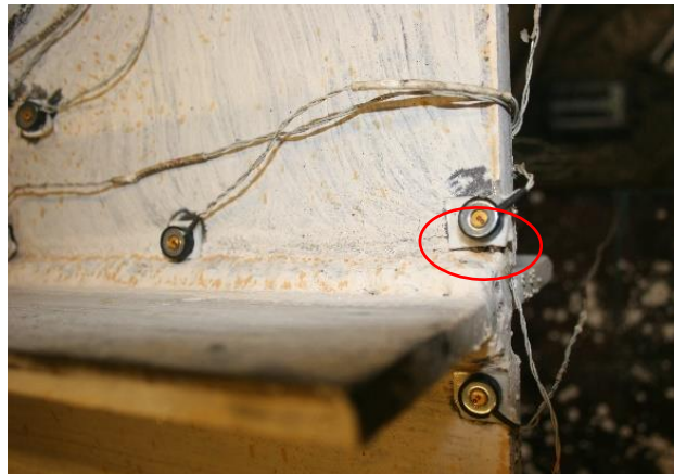
Figure 4.36 Beam Midspan Gusset Crack at Toe of Stiffener (N) 0.7%
