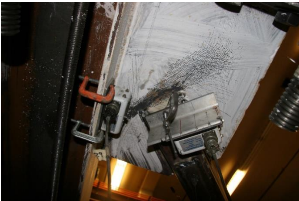
Figure 4.14 SE corner gusset @ +1.1%
