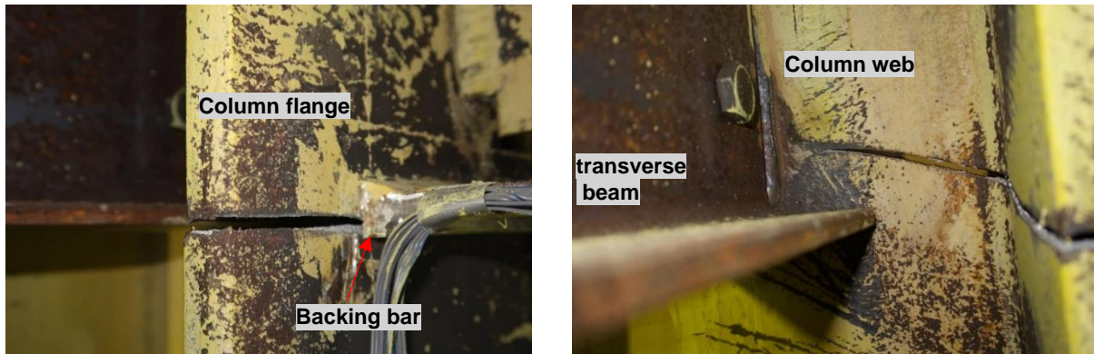
(c) fracture at backing bar
