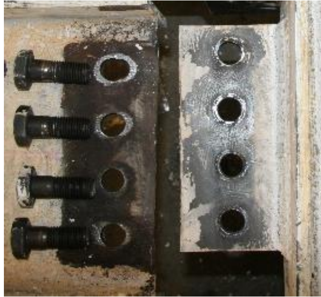
Figure 4.32 N Beam web bolt hole elongation
