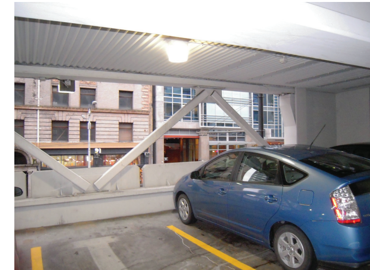
Figure 2.10: This garage at 1st Avenue and Pike Street has been seismically updated. Most existing garages in the CBD have not.
