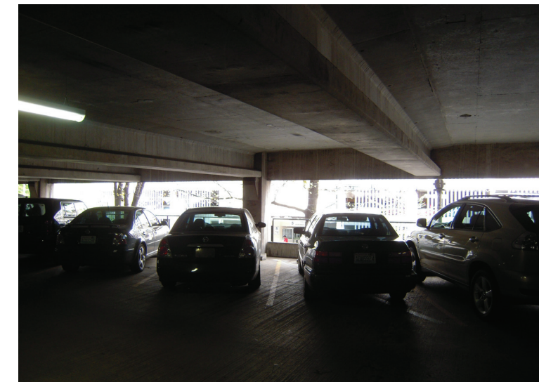
Figure 2.3: Concrete beams in two study garages with very low clearance to the underside of the structure
