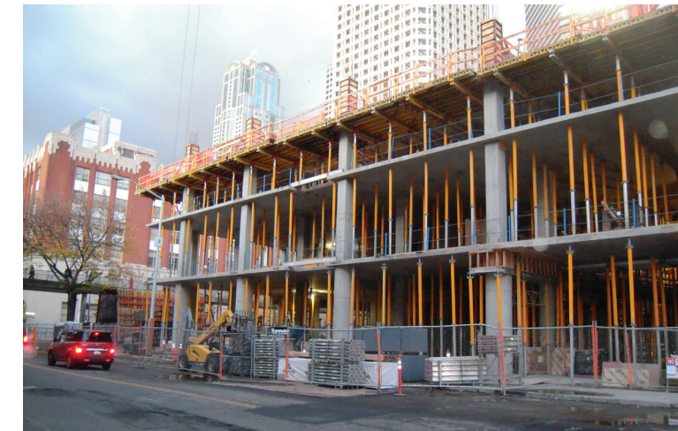
Figure 3.6: Comparison of the concrete structure of the existing Bon Marche garage (above) and the Colman Tower, a 16-story concrete frame building currently under construction (below), reveals constitutional similarity.
