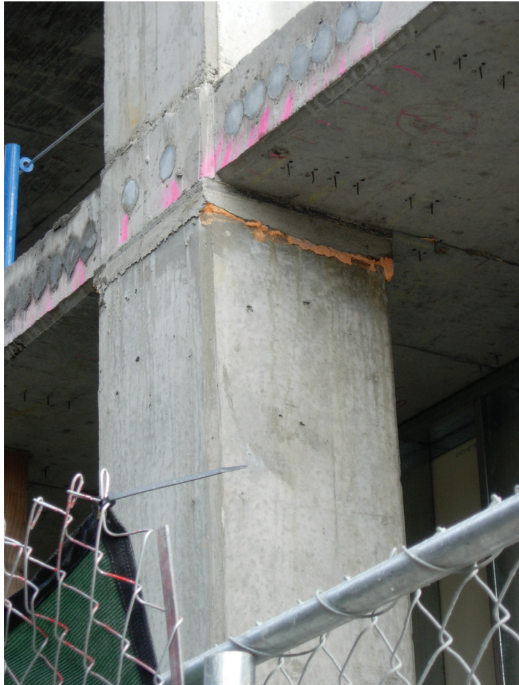
Figure 2.11: Capped steel tension cables at the exposed edge of a post-tensioned slab system under construction on the University of Washington's south campus
