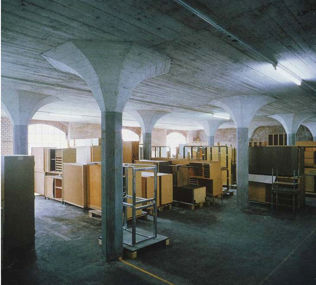
Figure 2.20 – Robert Maillart’s first “beamless slab”, Zurich Warehouse, 1910. (ARTstor Slide Gallery, Source: University of California, San Diego)
