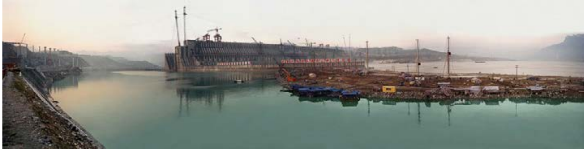
Figure 2.1: Panorama of the Three-Gorges Dam under construction. While China is the most recent nation to undertake such large scale water infrastructure projects, the legacy of these projects has shaped the Western United States Photograph By: Edward Burtynsky
