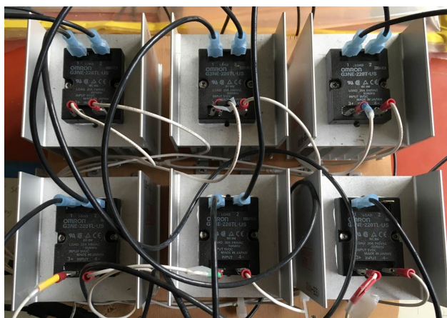
Figure A.8: Array of solid state relays for delivering power to heater elements. Software.
