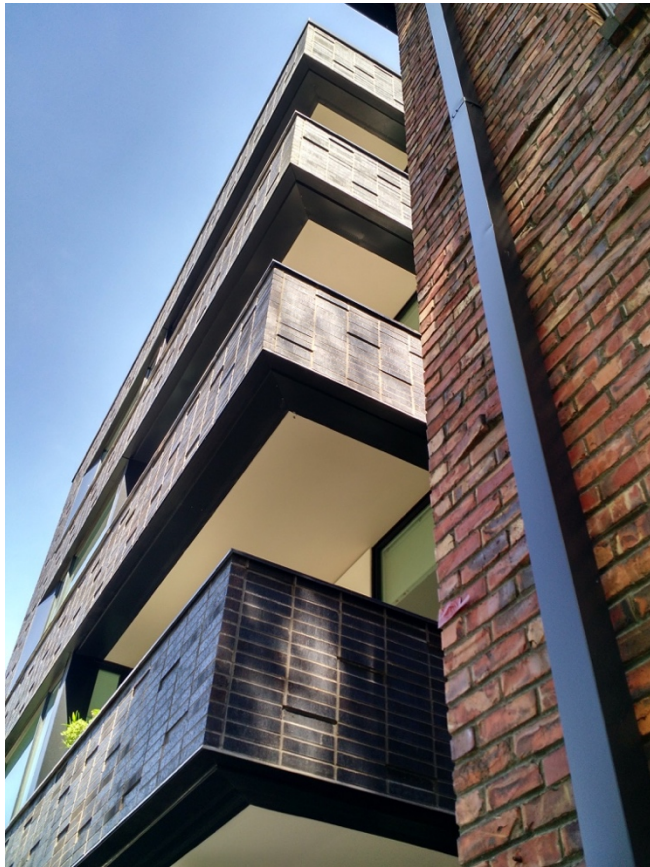
Figure 7 (at left): The balconies in question. Note the distressed brickwork on the addition, which was an attempt to complement the historic building at right. Source: Scott Cutler.
