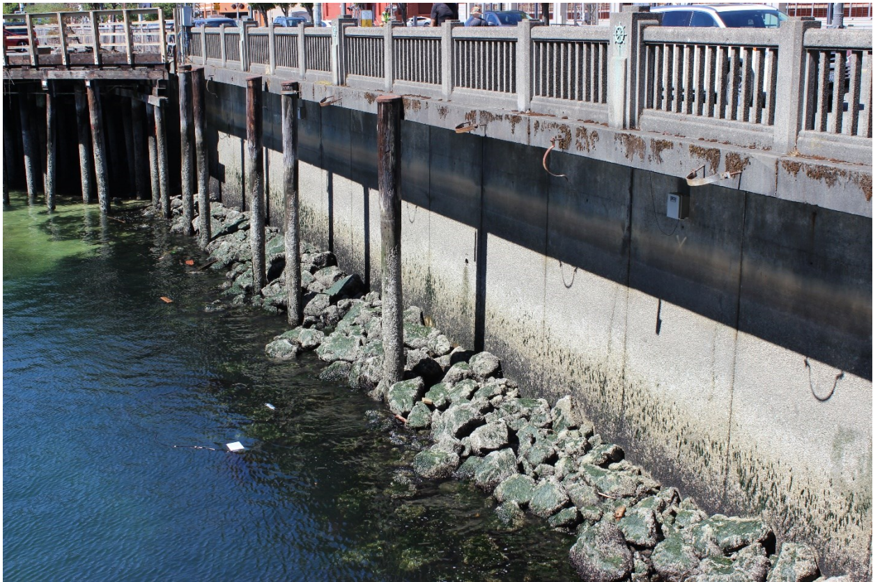
Figure 1. A section of the original flat concrete seawall fronted by rip-rap and a dark, shaded under-pier area in the upper left.
