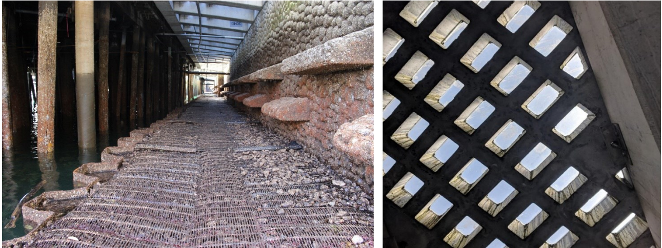
Figure 2. Seattle seawall eco-engineered enhancements. Left: In the foreground is the marine bench at low tide under a pier. On the right is the textured seawall with added shelves outside and under piers. Above are the cantilevered glass-paneled sidewalks (LPS). Right: View of LPS from below.
