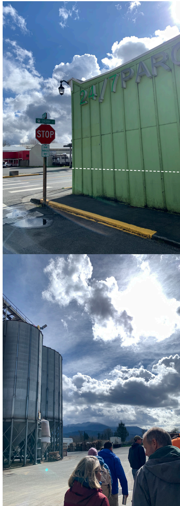
Figure 14. Top: Building with watermarks from November 2021 flood. Tour of private business.
