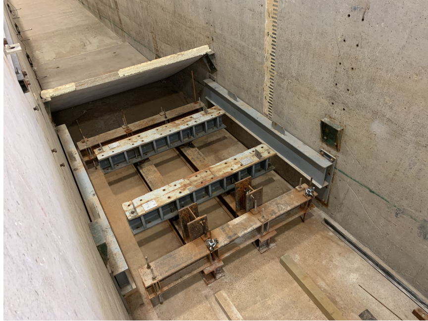
Figure 4.4: Reaction frame in base of flume
