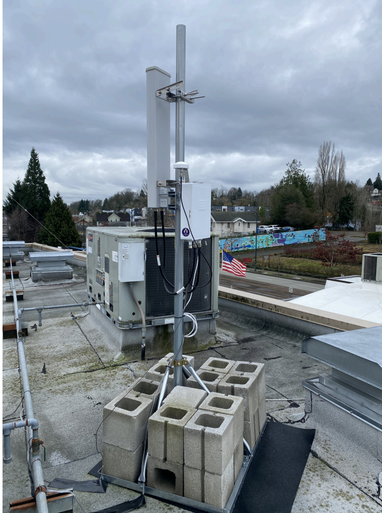
FCS Site Antenna Mast
