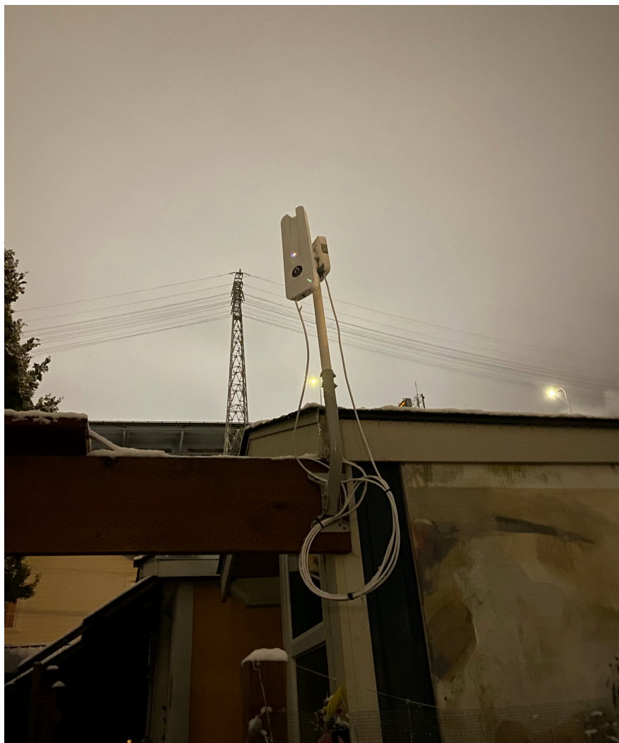
Northlake Village WiFi and PtP Equipment Mounted on Gate
