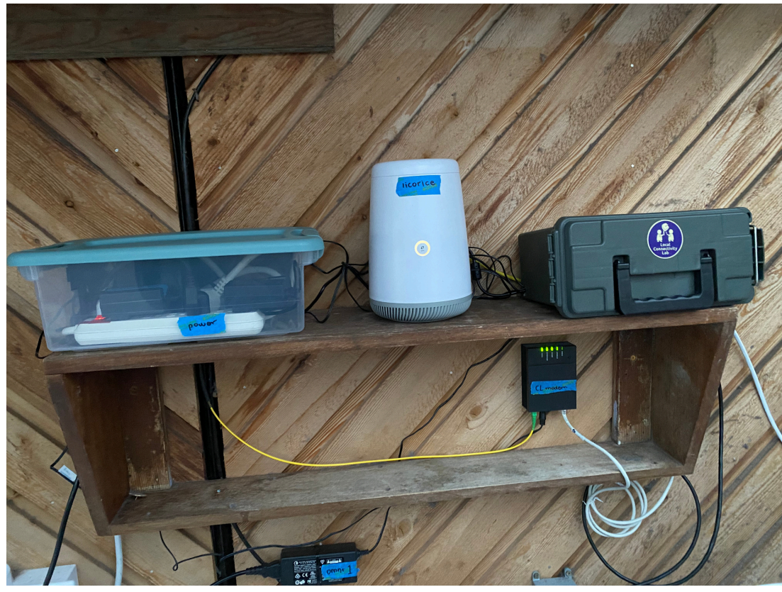
Lumen Fiber and SCN Equipment at Nickelsville CD Site After Fiber Upgrade
