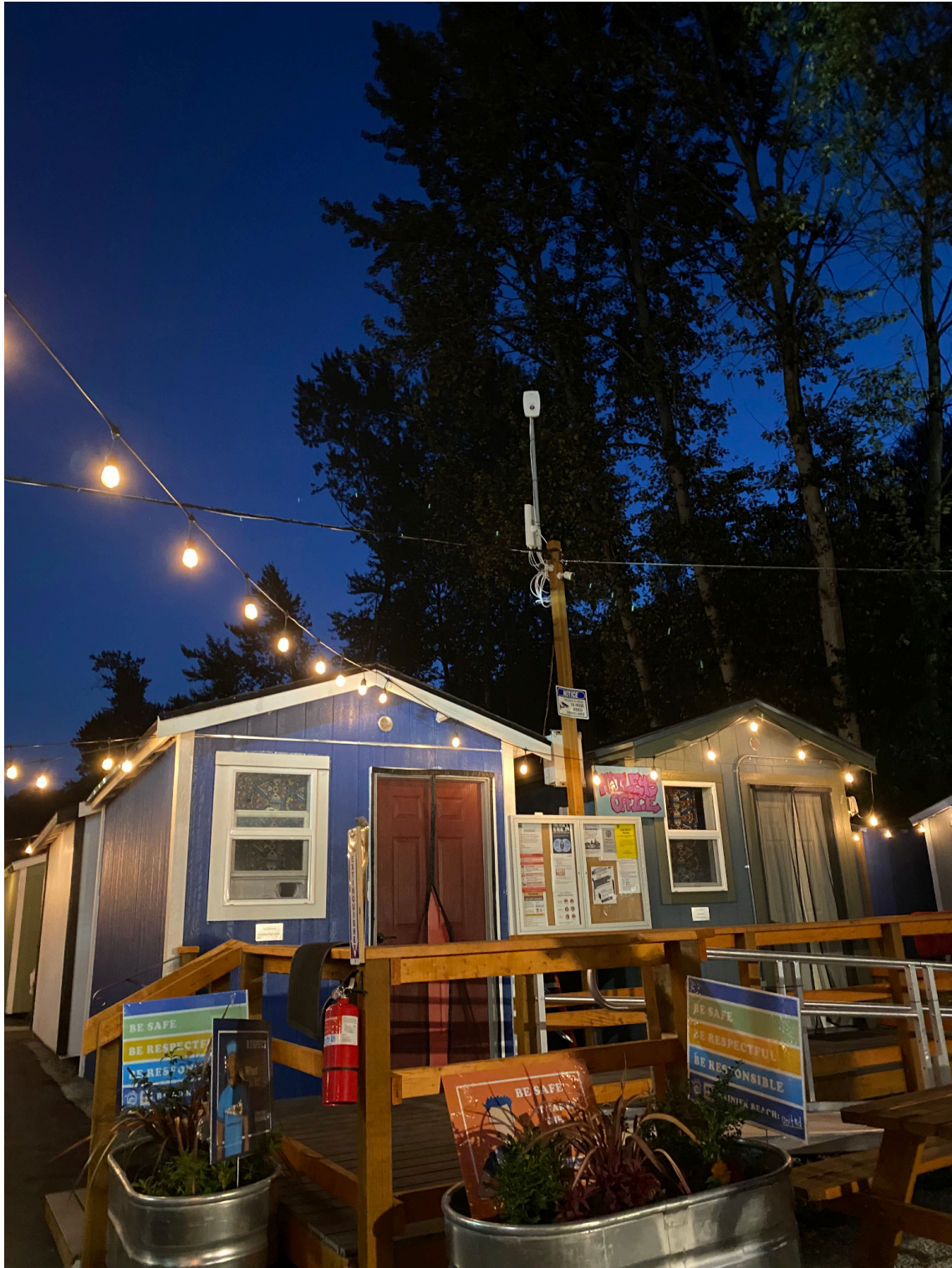
Network Equipment Installed at the Southend Village Site
