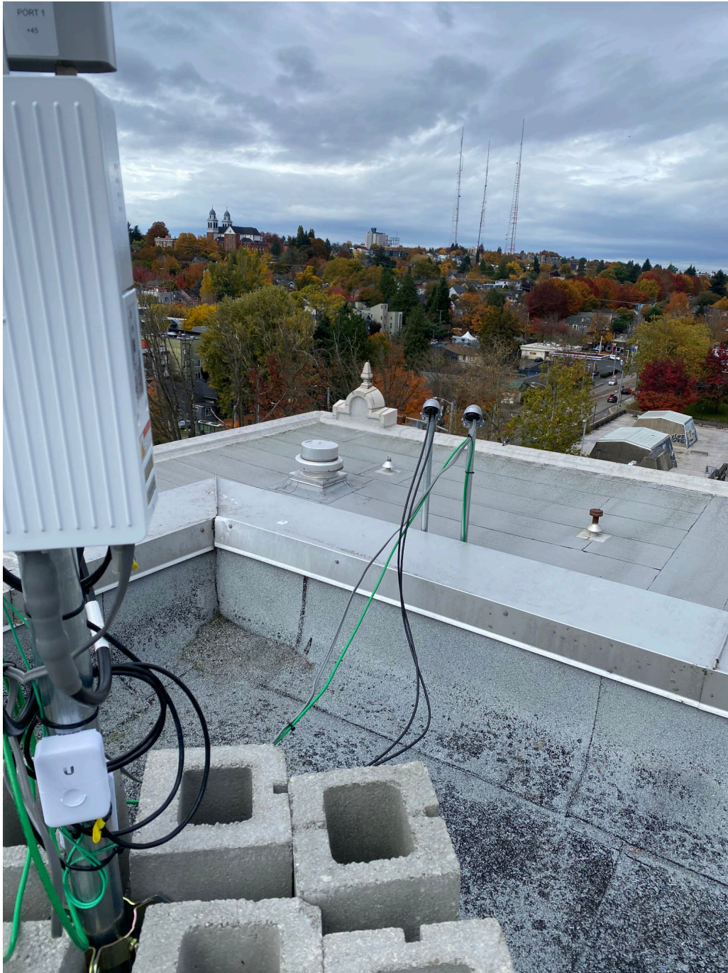
View from the Garfield High School Antenna Mast
