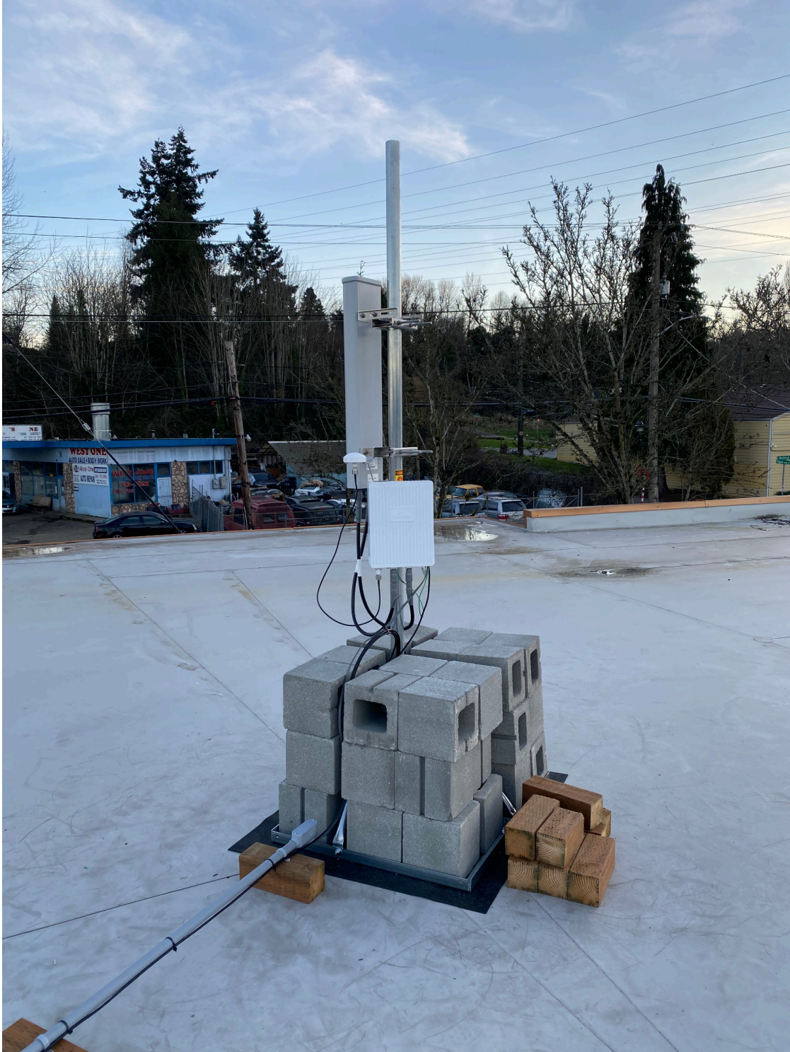
OCC Cell Site
