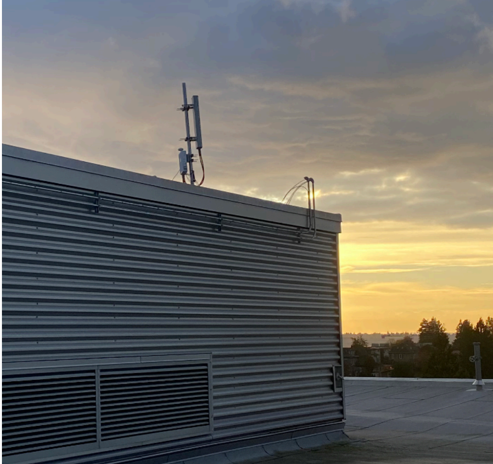
Fully Constructed Outdoor Antenna Mast at Garfield High School
