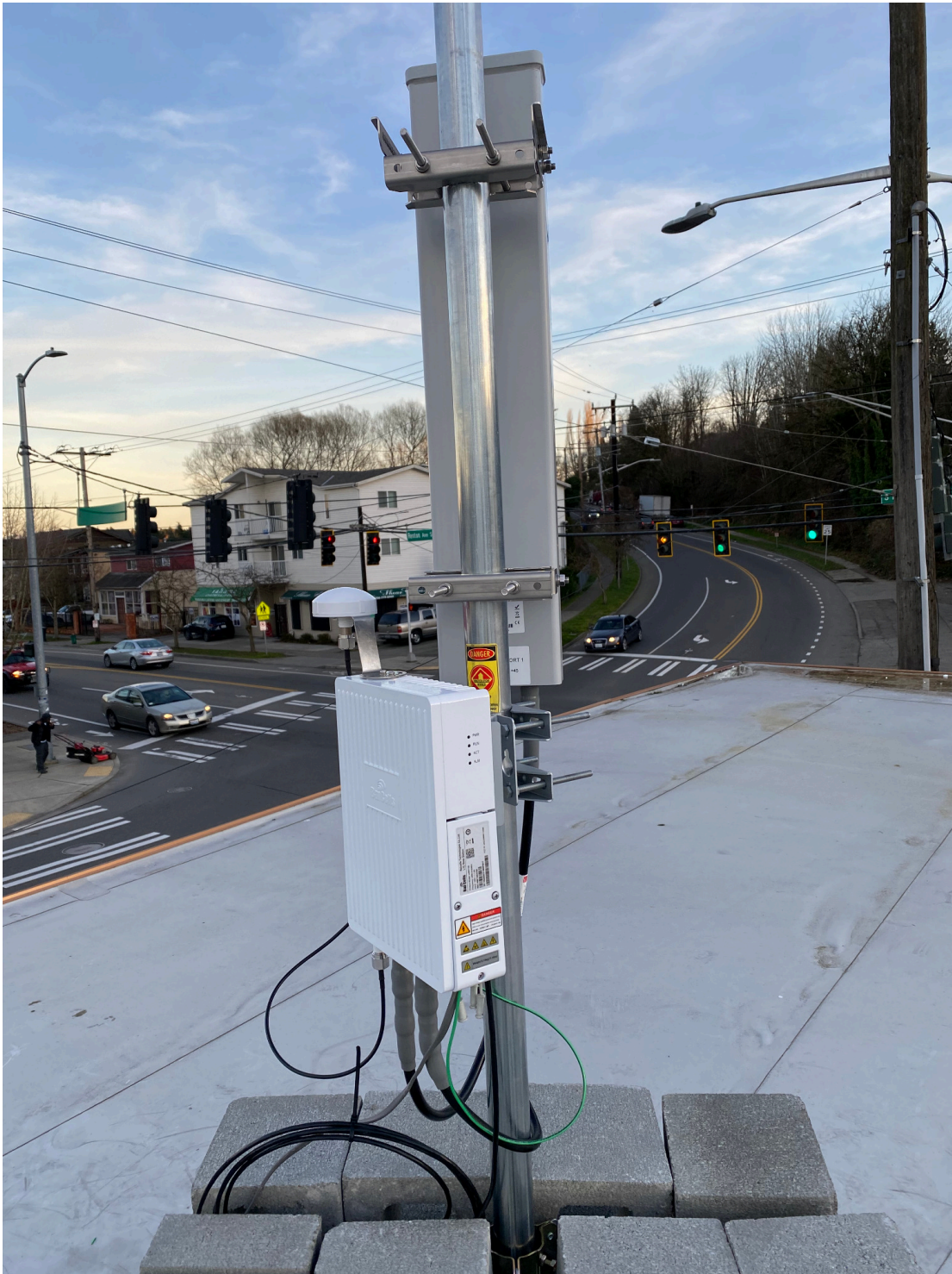
Close-up View of OCC Cell Site Antenna Mast
