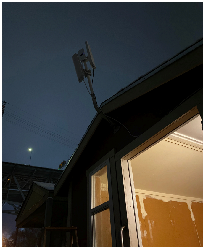
Northlake Village WiFi and PtP Wireless Equipment Mounted on Tiny Home
