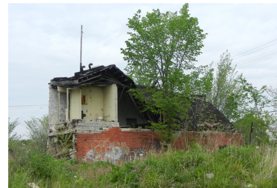
Figure 53| A burned and abandoned house.
