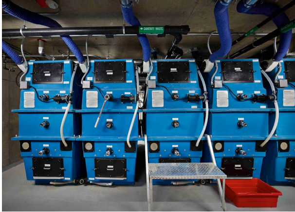
Figure 5 - Ten composting systems located in the basement of the Bullitt Center
