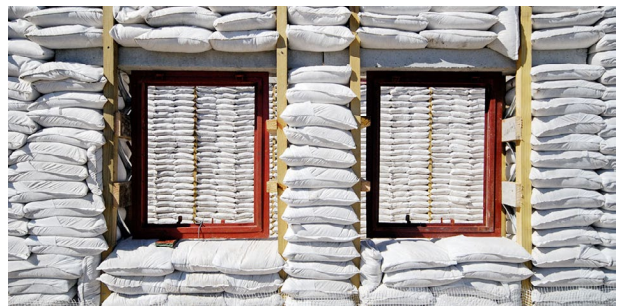
Figure 9 - A construction view of two window frames showing the placement and density of the sandbags.
