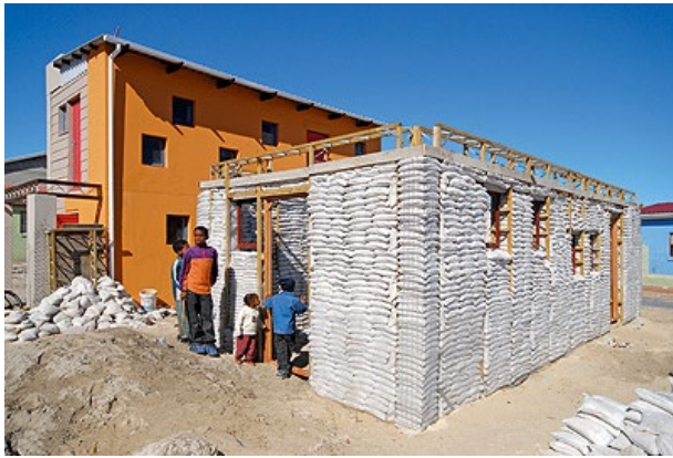
Figure 8 - A construction view of a house showing the placement and density of the sandbags.
