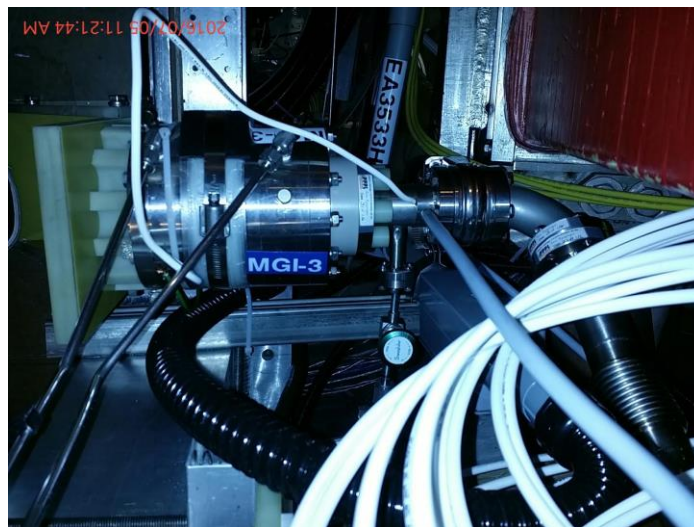
Figure 3.3. The final version of one of the three MGI valves installed on NSTX-U. A total of three valves are installed on NSTX-U. Two valves are fully operational.
