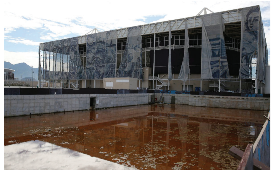
Figure 28: The aquatic center was supposed to be divided into community pools but instead is tattered and in disrepair. The standing water in the pools is not safe for people to swim in.
