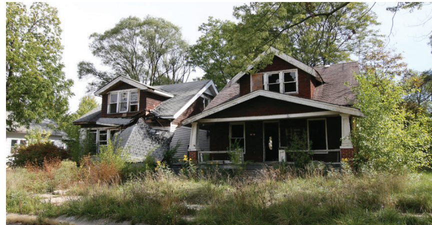
Figure 48: The blight often found in Detroit neighborhoods manifests in overgrown yards, collapsing homes, and fire-damaged structures.
