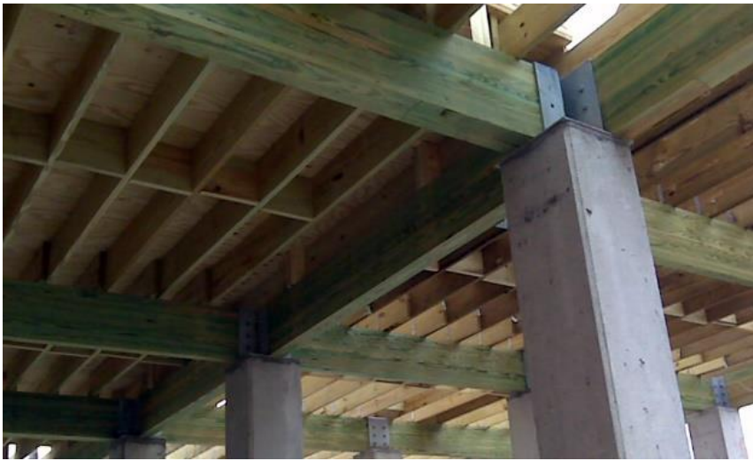
Figure 4-4 Glulam Beam on Precast Concrete Column Carrying Floor Load (Source: Anthony Forest Products)
