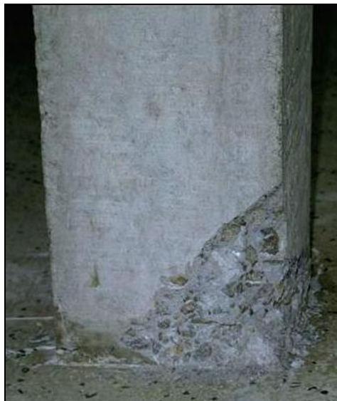
Figure 3.40 Concrete spalling on flexural and side face: earthquake damage (PEER)
