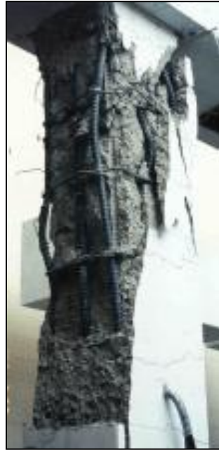
Figure 3.99 Crushing of core concrete: experimental damage (Sezen 2002)
