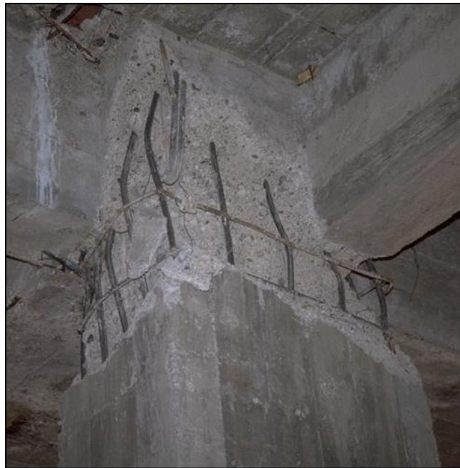
Figure 3.54 Crushing of core concrete: earthquake damage (PEER)
