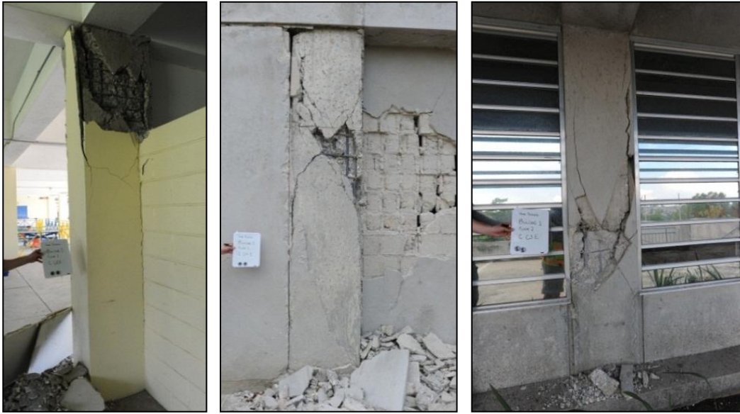
Figures 3.84, 3.85, and 3.86 Concrete spalling on side faces: earthquake damage (Eberhard, et al. 2010)
