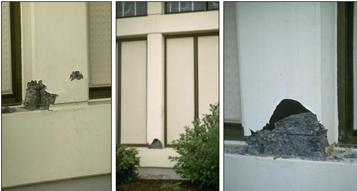
Figures 3.44, 3.45, and 3.46 Concrete spalling exposing longitudinal steel: earthquake damage (PEER)
