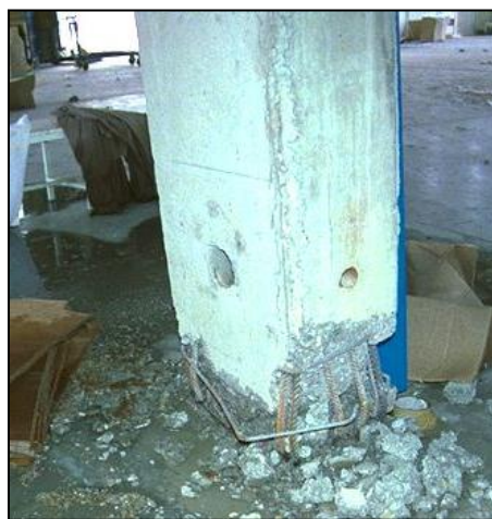
Figure 3.50 Longitudinal bar buckling: earthquake damage (PEER)
