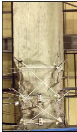
Figure 3.13 (F5) Concrete Spalling Exposing Longitudinal Steel
