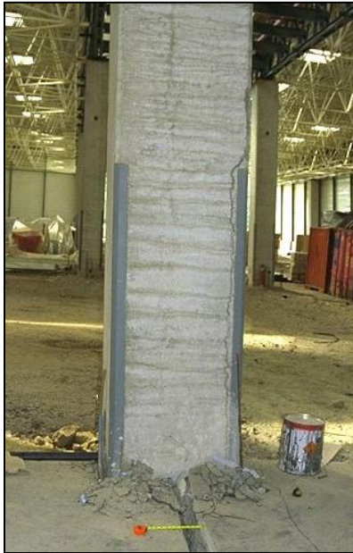
Figure 3.35 Longitudinal cracking: earthquake damage (PEER)
