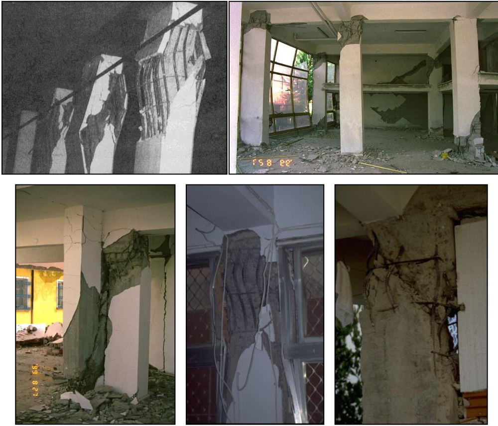
Figures 3.92, 3.93, 3.94, 3.95, and 3.96 Longitudinal bar buckling: earthquake damage (PEER)
