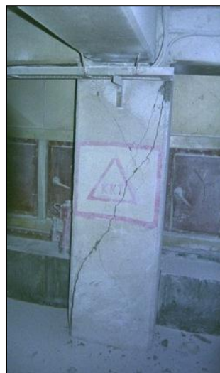
Figure 3.73 Widening and localization of shear cracks: earthquake damage (PEER)
