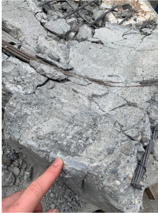
Figure 7-25. Grooves from epoxy mortar where pile-column wall slipped
