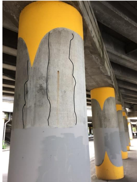
Figure 1-2. Longitudinal cracks on columns of Ravenna Bridge
