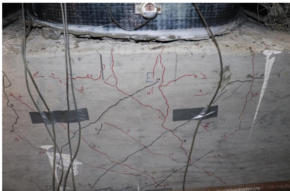
Figure 7-5. Progressive joint shear cracking on base beam on Series 8 (+4.70%, -5.49% drift)
