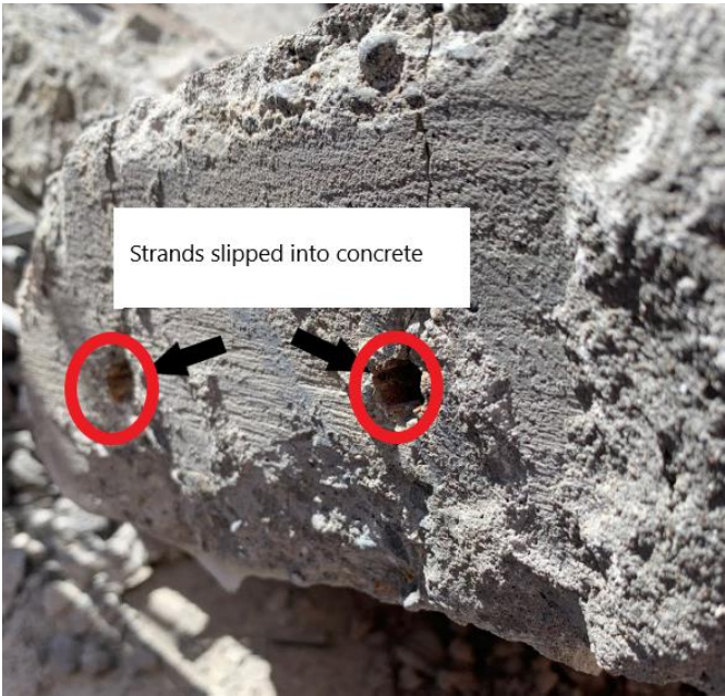
Figure 7-22. Slipped strands at base of pile-column wall
