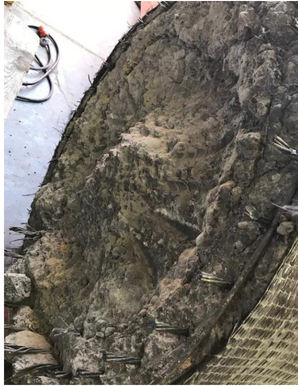
Figure 7-19. Top segment of specimen after detachment from plug connection to cap beam
