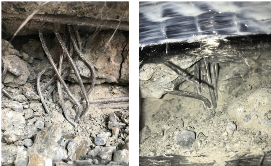
Figure 7-16. Buckled strand (left) and fractured strand (right)
