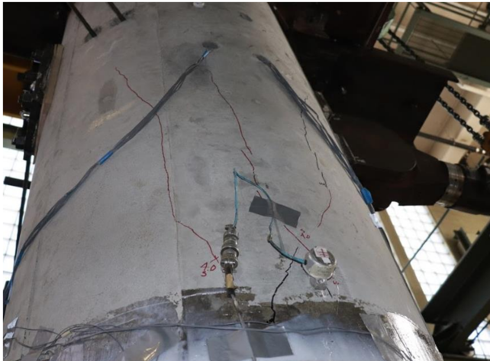
Figure 7-8. Progressive cracking above fiber on Series 8 (+4.71%, -5.49%)
