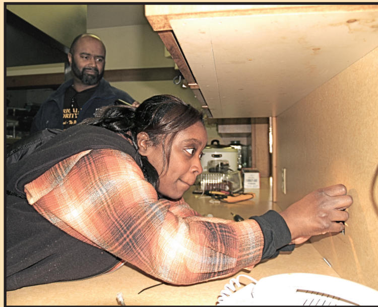
Electricians Felicia Wiseman of IBEW Local 58 in Detroit and Jeff Thomas of IBEW Local 11 in Los Angeles troubleshoot electrical outlets at the Salvation Army in North Portland. Union electricians attending the National Conference of Electrical Workers Minority Caucus in Portland Jan. 14-18 fanned out across the city on Jan. 14 for a "day of service," in observance of the Martin Luther King Jr. holiday. The Salvation Army received new electrical receptacles in the kitchen and gymnasium, old and non-functioning receptacles were replaced, new circuits were added to the main circuit panel, and all circuits in the main panel were matched to their proper receptacles and locations in the building.
