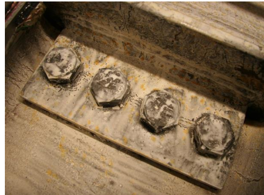
Figure 4.10: Initial shear tab yielding at -1.1\% drift (Y1).
