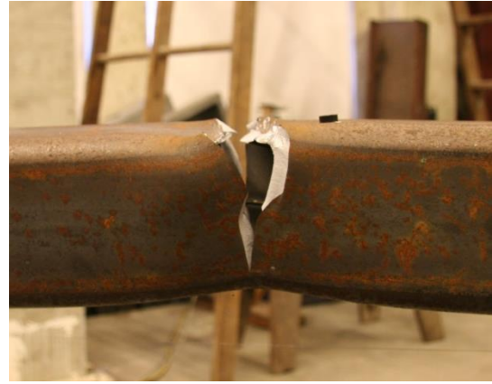
Figure 4.83: N brace \frac{3}{4} tear at -3.3% drift (B3-BT).
