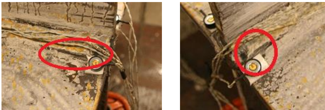
Figure 4.21: Plate cracking at S (left) and N (right) gusset-to-stiffener welds (PC1).
