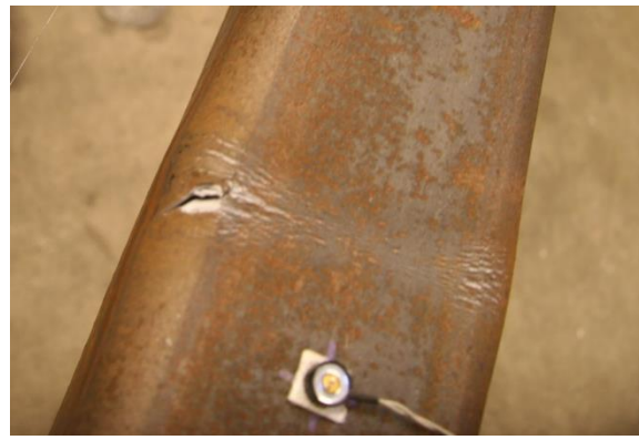
Figure 4.81: N brace crack/striations at -3.3% drift.
