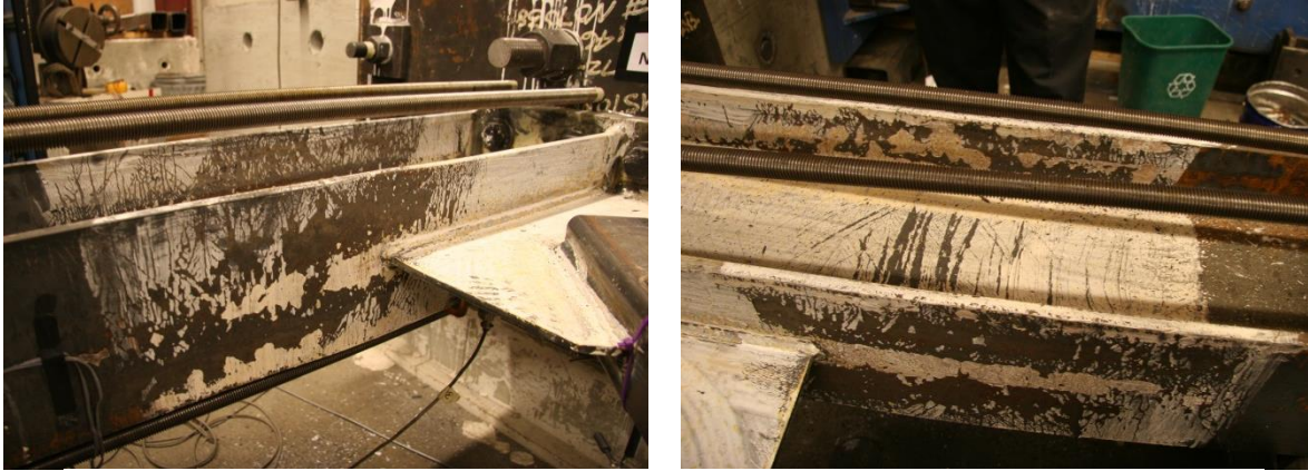
Figure 4.22: Severe yielding in N col. (left) and S col. (right) at 2.76% drift (Y3-PH).
