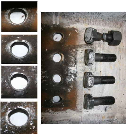
Figure 4.28: S beam web bolt hole elongation.
