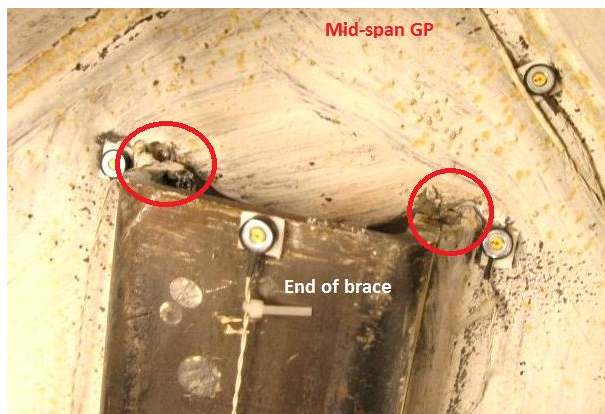
Figure 4.48: Plate cracking at toe of brace-to-mid-span gusset weld (PC1).
