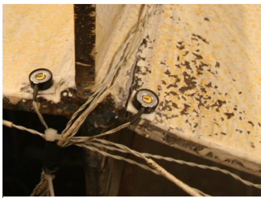
Figure 4.80: Plate crack at N mid-span gusset-to-stiffener weld at 3.3% drift (PC2).
