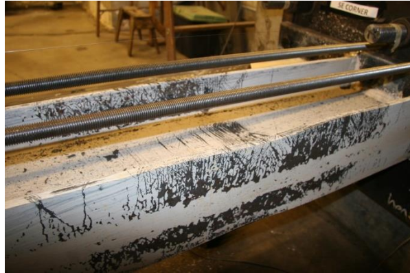
Figure 4.77: S col. severe yielding at 2.8% drift (Y3-PH).
