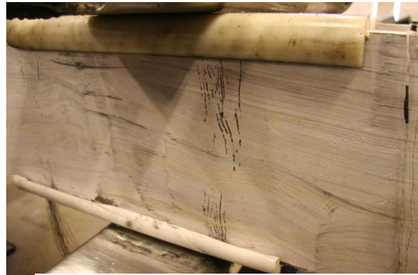
Figure 4.38: Beam OF initial yielding at 1.4\% drift (Y1-OF).
