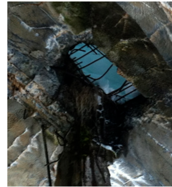
Degraded roof slab 30. South end of shed showing 31. run-off paths above Collapse at south end 32.
