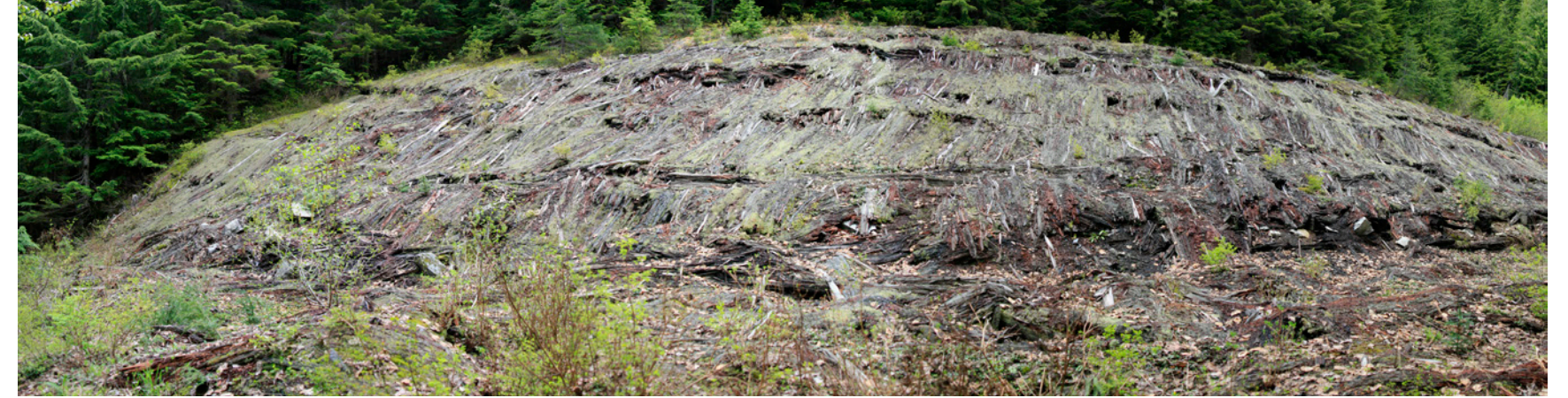
25. Collapsed wood snow shed
