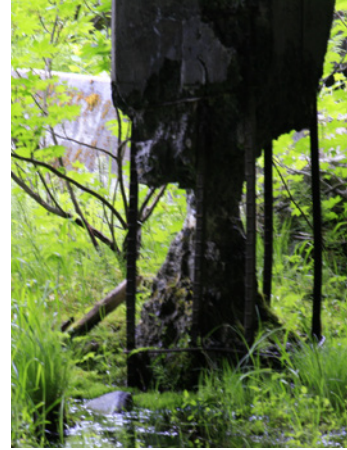
Degraded concrete column 22. Historic wood cabins 23. Sheet metal in the landscape 24.
