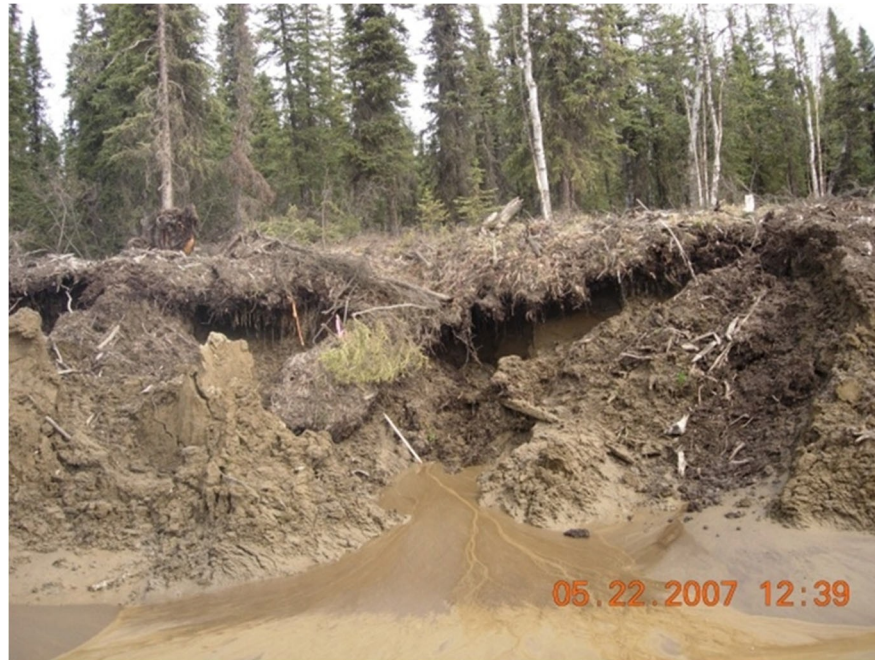
Figure 6-3 Advanced thaw degradation of a cut slope shows block failures and runoff of highly fluid silt into a ditch
