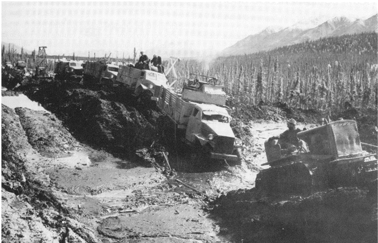
Figure 1-1 Thawing permafrost during the construction of the Alaska-Canadian Highway (Coates 1982).
