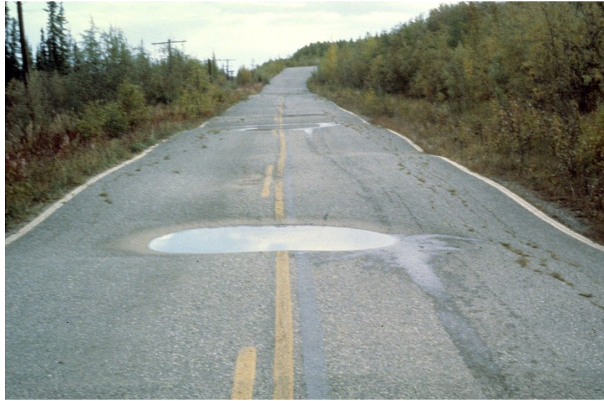
Figure 1-3 Roadway damage on an abandoned section of the Richardson Highway east of Fairbanks (photo B. Connor)
