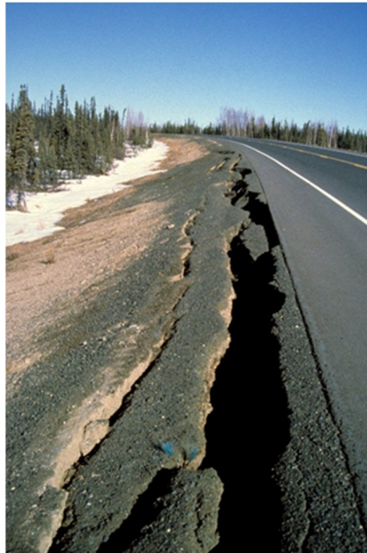
Figure 7-6 Longitudinal cracking due to thawing permafrost (photo DOT&PF)
