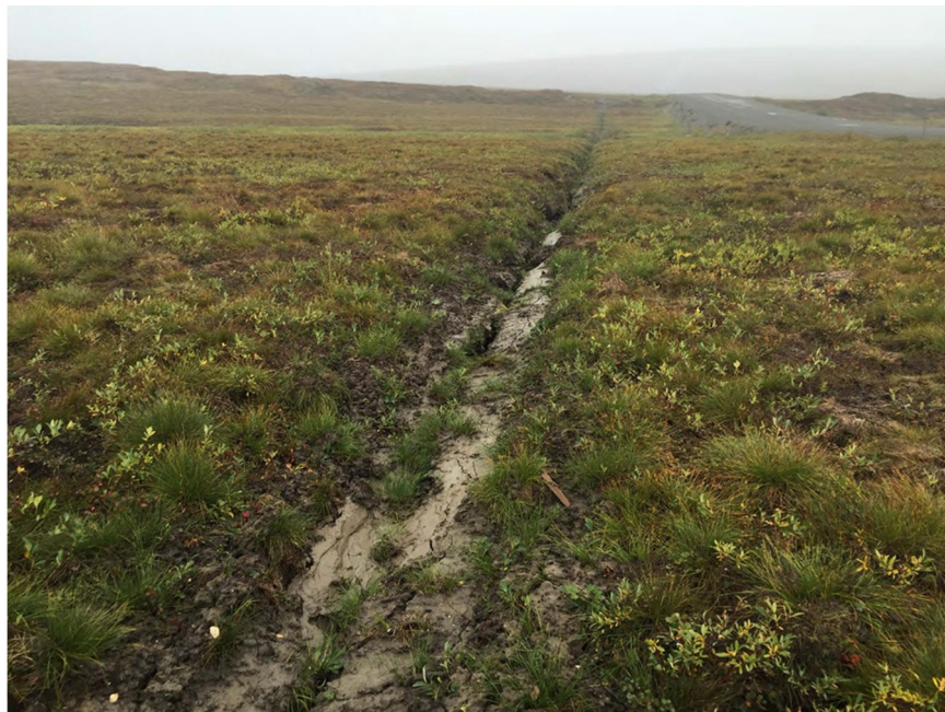
Figure 7-2 An example of advection along the Dalton Highway from the installation of fiber optic cable. Photo by Mikhail Kanevskiy
