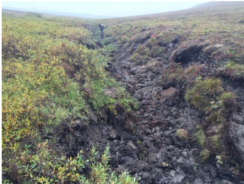
Figure 7-3 Erosion due to advection resulting from installation of fiber optic cable along the Dalton Highway. Photo by Mikhail Kanevskiy
