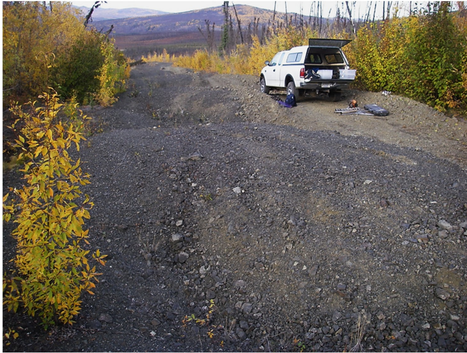
Figure 2-9 Thermokarst mounds (baydzherakhs) developed because of ice-wedge degradation under the abandoned part of the Dalton Highway, interior Alaska.
