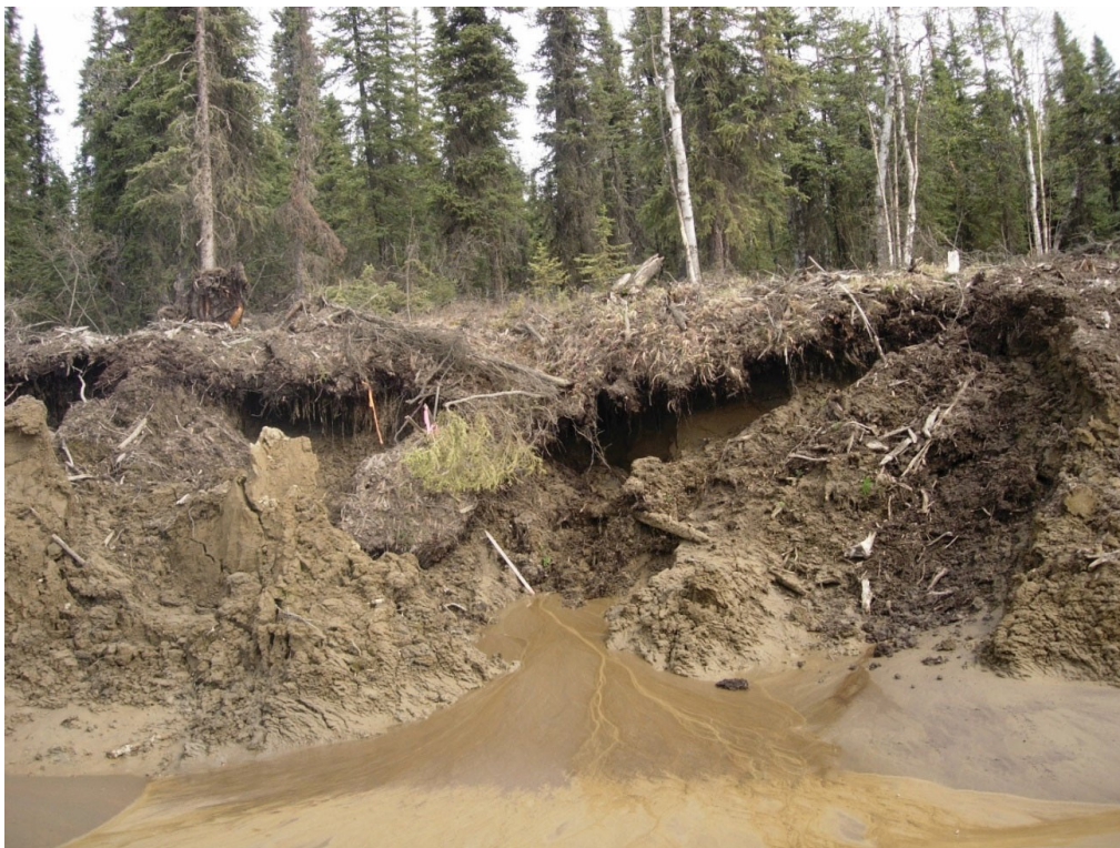
Figure 1-2 Thawing permafrost slopes along the Dalton Highway (photo by DOT&PF)
