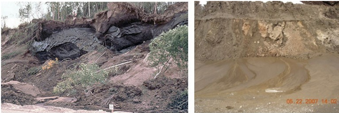
Figure 6-2 Massive ice exposed in a cut slope (left) and runoff from a thawing ice-rich cut slope (right).
