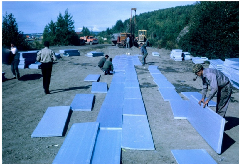
Figure 5-4 Installation of DOW extruded foam insulation at Fairhill Road near Fairbanks, Alaska
