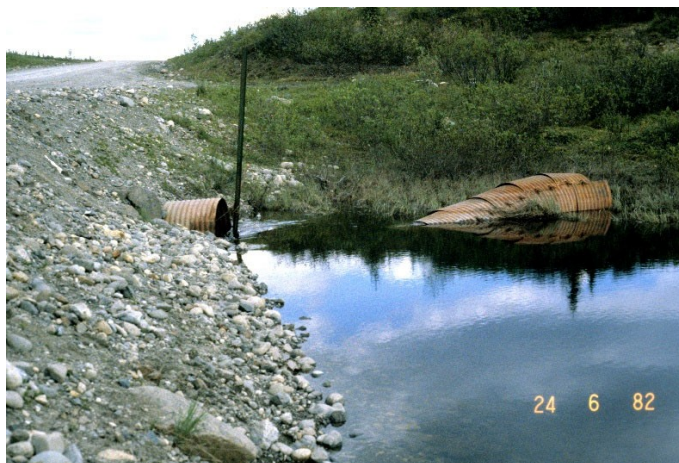
Figure 7-12 Settlement of an inlet due to advection
