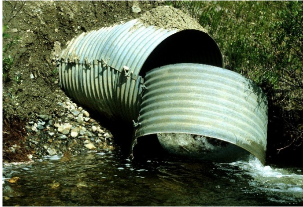
Figure 7-10 Erosion at the toe of slope due to advection
