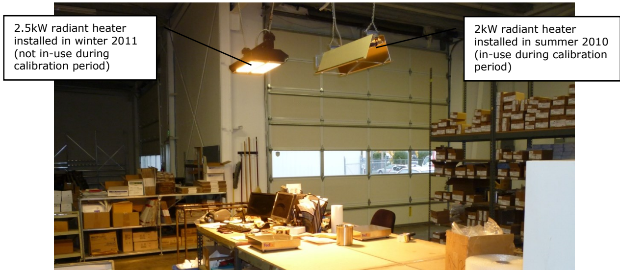
Figure 79 - Picture of radiant heaters mounted over the E Warehouse packing area
