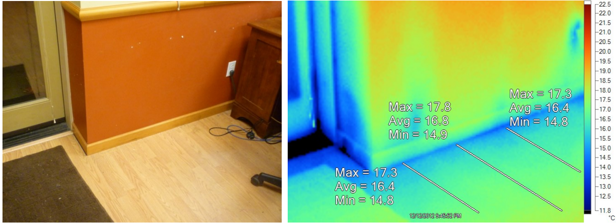
Figure 72 - Thermal and photo images of Office floor at north wall
