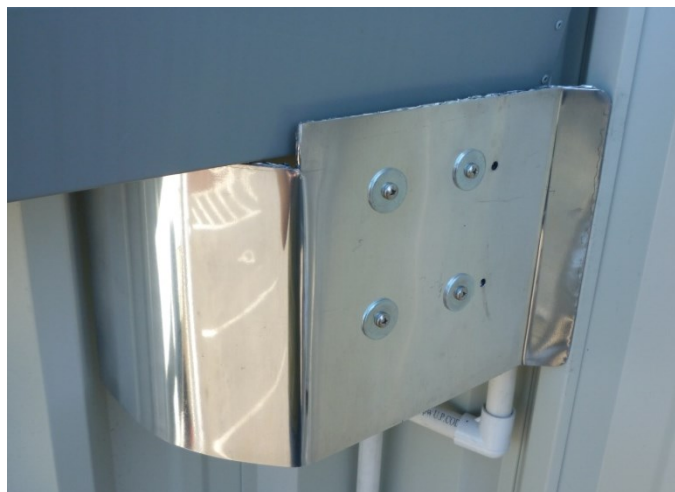
Figure 17 - Close-up of custom outdoor air temperature shield
