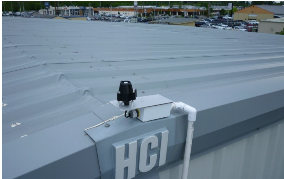
Figure 10 - Solar radiation sensor installed on the roof
