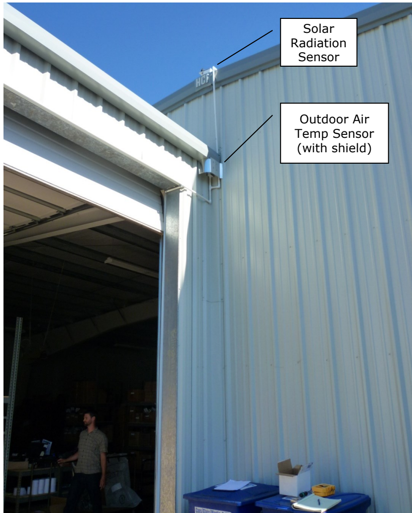
Figure 16 - Outdoor air temperature and solar radiation sensor location
