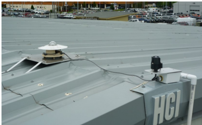
Figure 34 - Photo of installed Davis and Eppley global solar radiation sensors
