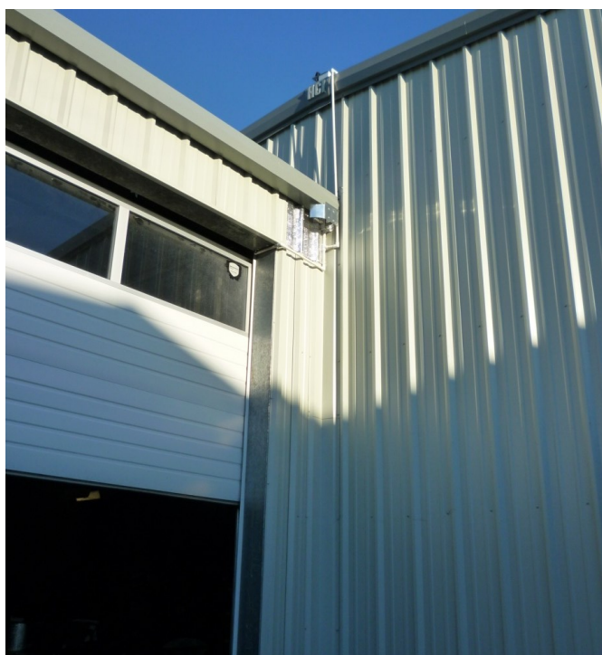
Figure 40 - Photo of building OADB sensor in direct sun, observed for short periods of each afternoon evening.
