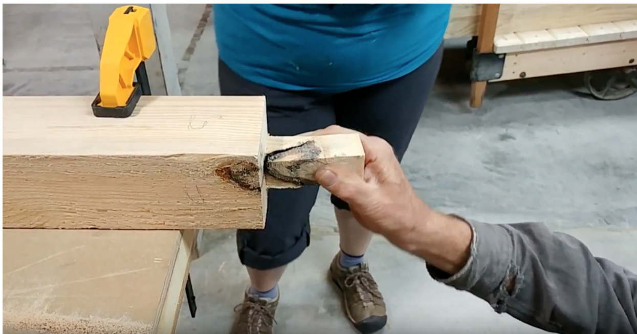
Figure 3: Helen finds a knot when carving this tenon for a wall stud. The knot's placement meant the tenon would not be strong enough, so this piece was reused for another purpose.
