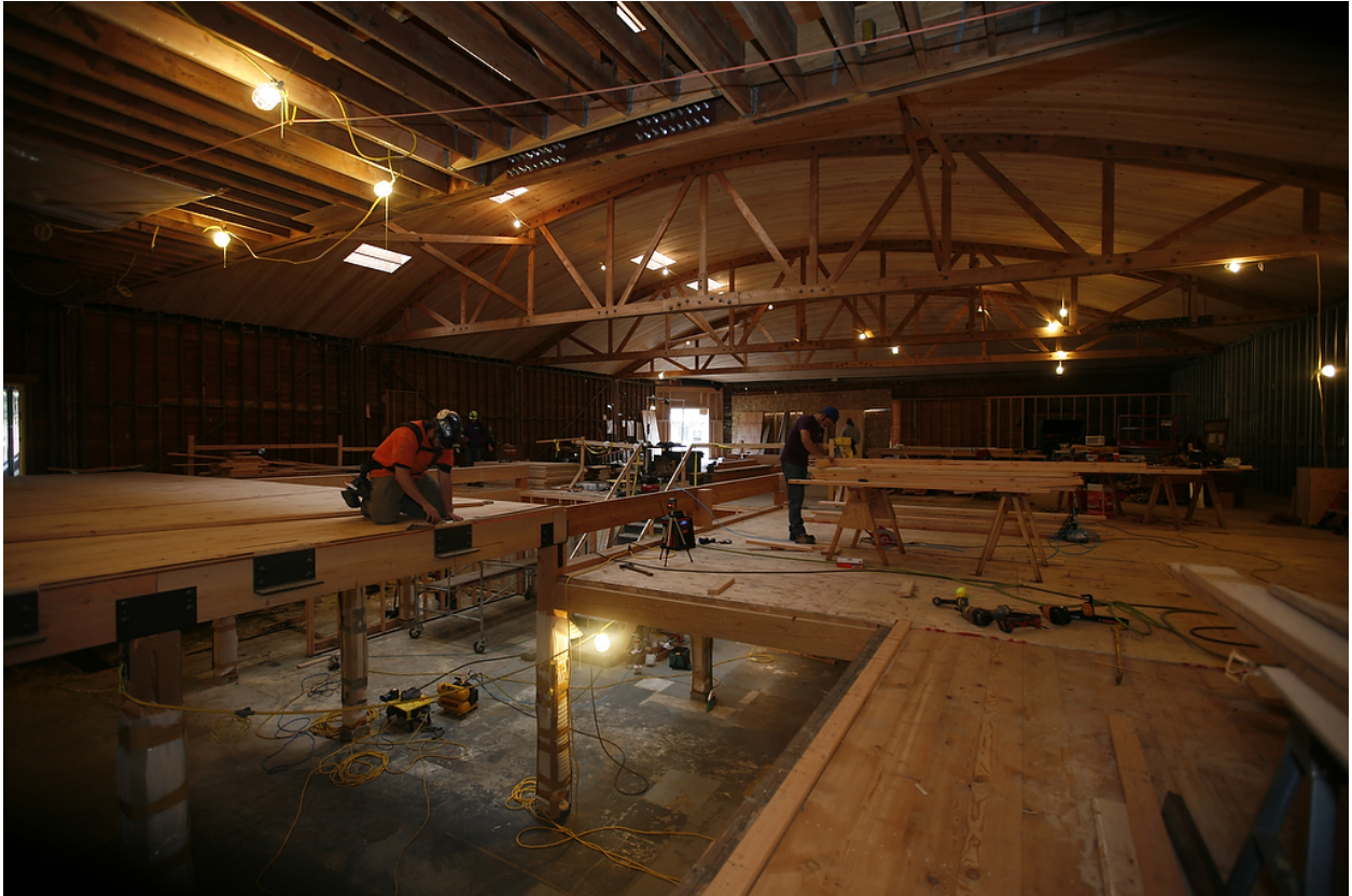
Fig. 43: The renovation of the old Thriftway was substantially extensive, involving removing the existing false ceiling and floor, as well as cutting new window openings on the north wall. Much of the interior character, or lack thereof, was removed. (Métis Construction)
