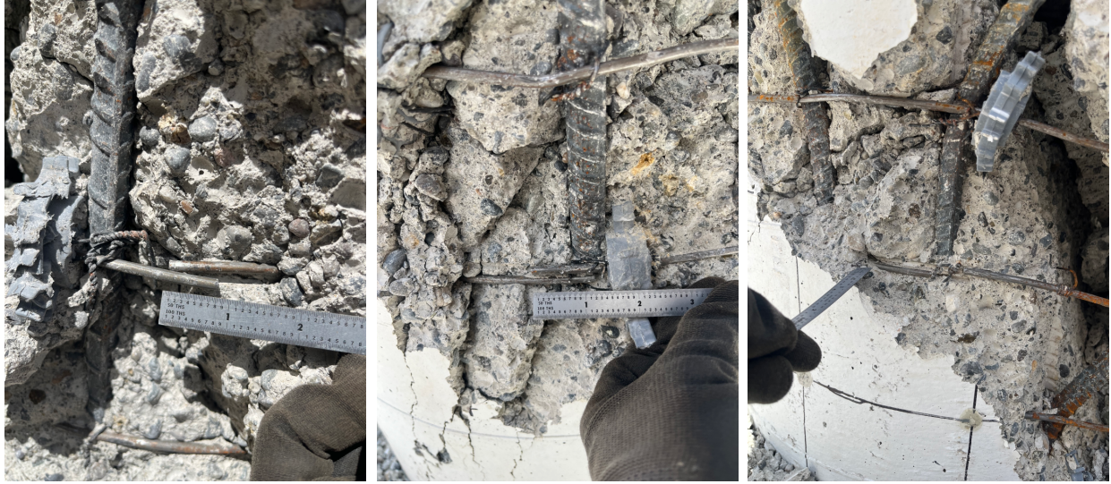
Figure 5.4 Final state of overlapped ends in hoops after clear cover removal, showing a reduction in length (initially was 4 in.)
