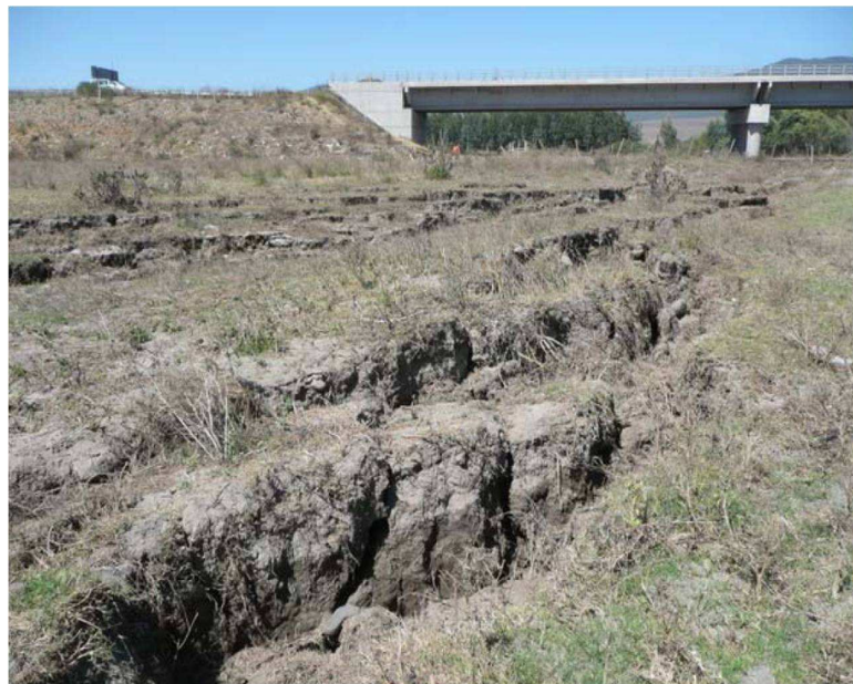
Figure 6.1: Lateral spreading on northern river bank at Puente Mataquito as seen from ground surface (GEER, 2010a).
