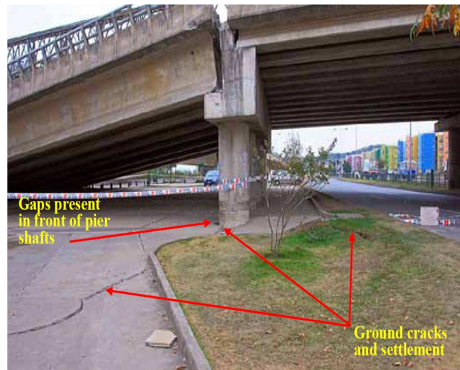
Figure 6.3: Portion of northeast approach to Puente Llacolén affected by liquefaction-induced ground deformation (FHWA, 2011).
