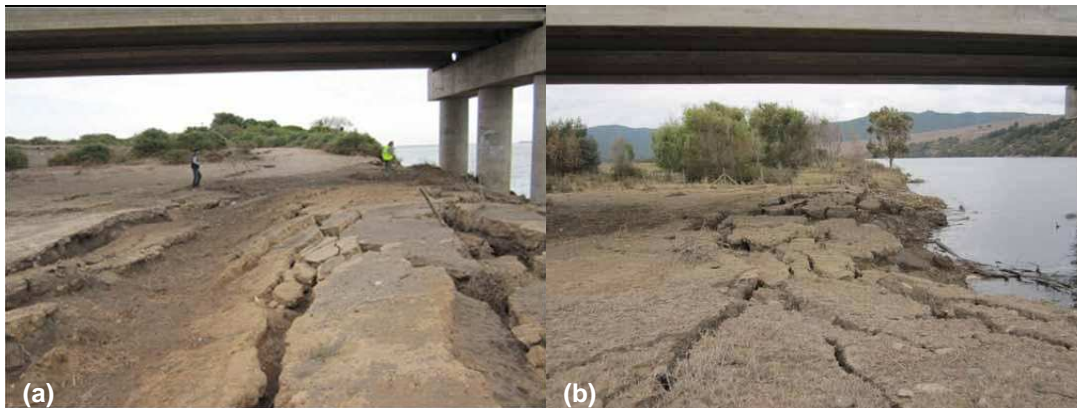
Figure 6.7: Surface manifestation of lateral spreading at Puente Mataquito. (a) Southwest approach (GEER, 2010a). (b) Northeast approach (MAE, 2010).
