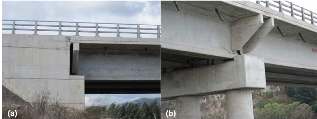
Figure 6.8: Minor structural damage caused by lateral spreading (GEER, 2010a). (a) Crushing of NE abutment. (b) Shearing of bridge girder above interior piers.
