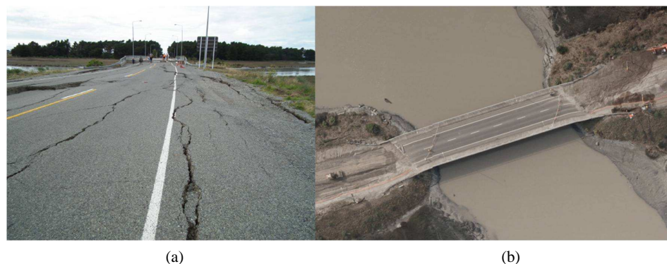
Figure 1.5: South Brighton Bridge after the Christchurch event. (a) Longitudinal lateral spreading cracks in western approach embankment (Cowan, 2011). (b) Aerial photo with visible lateral spreading cracks on river banks (LINZ, 2011).
