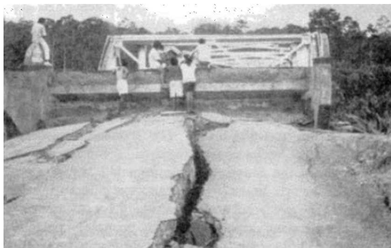
Figure 1.3: Settlement and longitudinal cracking of southern approach embankment at Rio Estrella Highway Bridge (Youd, 1993).
