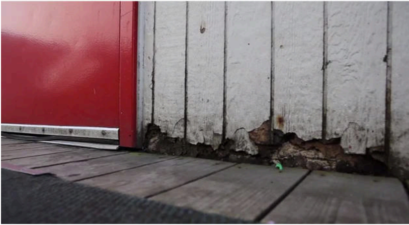
Figure 2.1 - siding rot on modular classroom, Bellingham, WA
