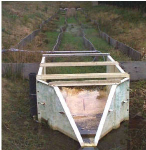
Figure 3.3. Two-foot H-flume at Pine Lake outlet.
