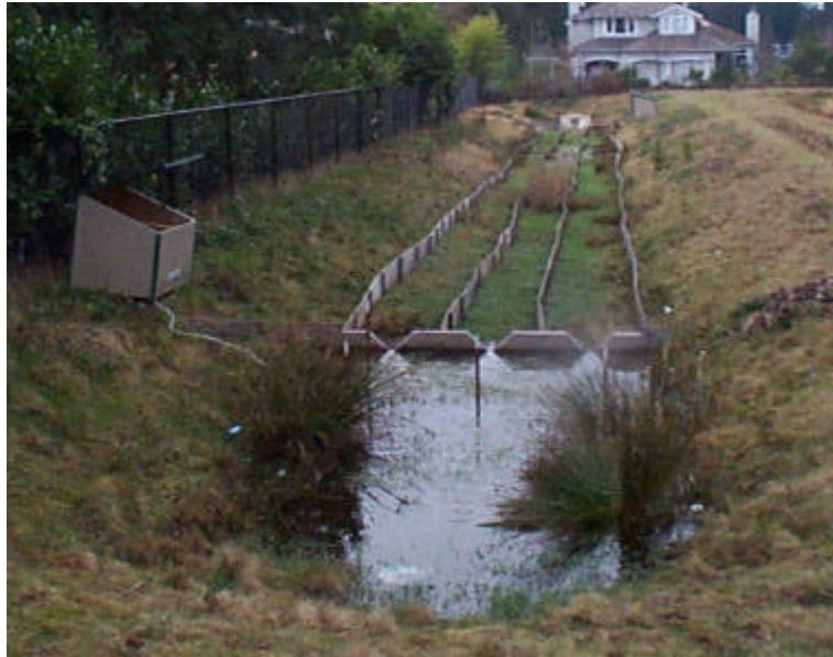
Figure 3.1. Pine Lake swale divided into three channels. Channel designations (from the left) PL1, PL2, and PL3.
