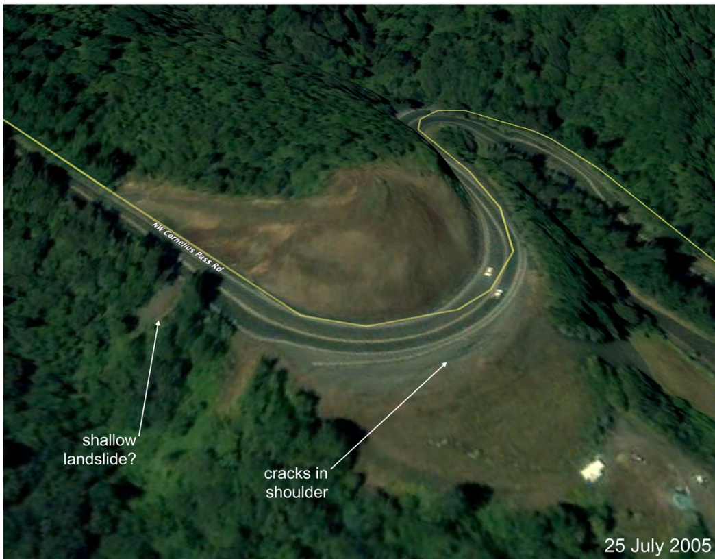
Figure A2.2.3. Shallow landslide between 2002 and 2005. Cracks have begun to develop in the shoulder
