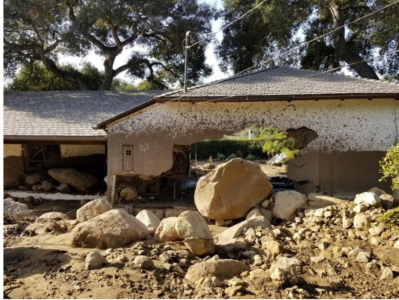
Figure A2.5.2. Home violently destroyed by the January 2018 Montecito, California, debris flow. Image: Kean et al. (2019b)
