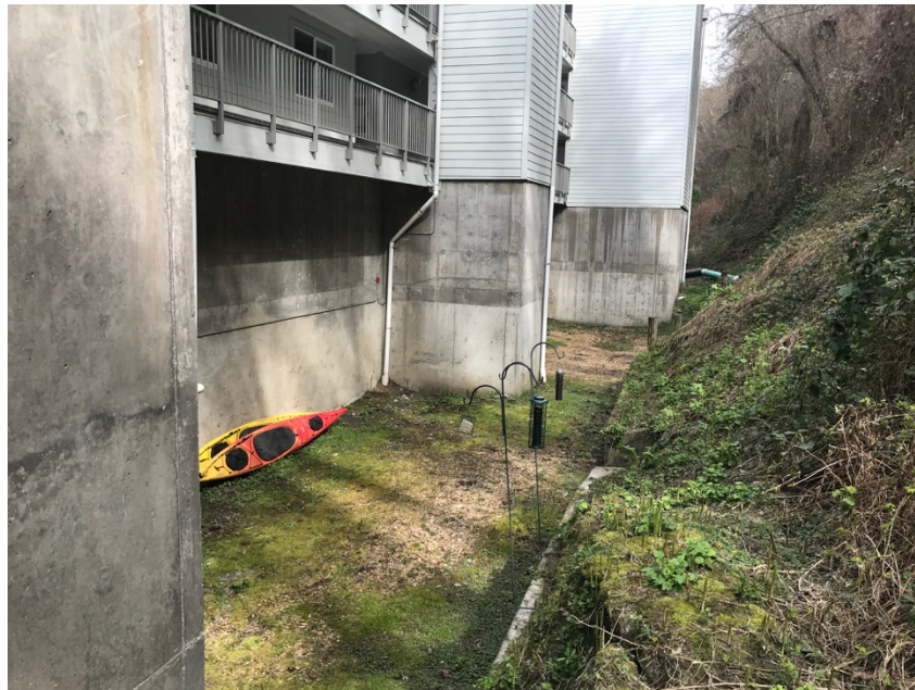
Figure 6.31. An apartment building along Alki Avenue with a reinforced rear wall. A landslide overran the low concrete block wall in the center of the image and struck the building, leaving mud splash marks up to 8 ft high (above the kayaks). The undisturbed portion of the deposit is on the right side of the image.
