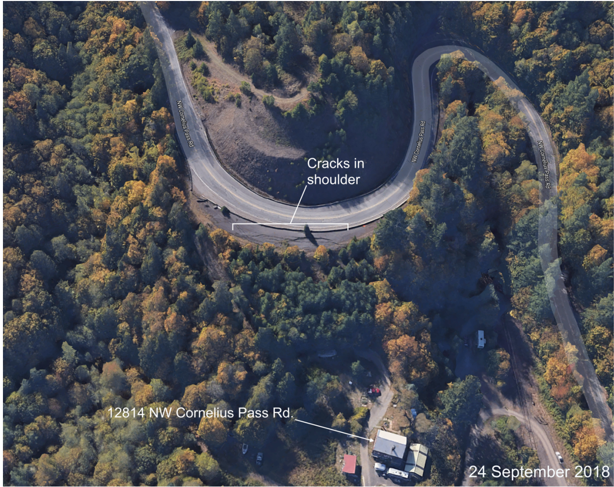
Figure A2.2.5. Well developed cracks in the shoulder and pullout above 12814 NW Cornelius Pass Rd. suggesting ongoing deep-seated slope deformation.
