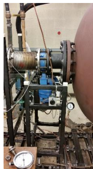
Figure 2.2. Butterfly valve (in blue) set upstream of dump tank
