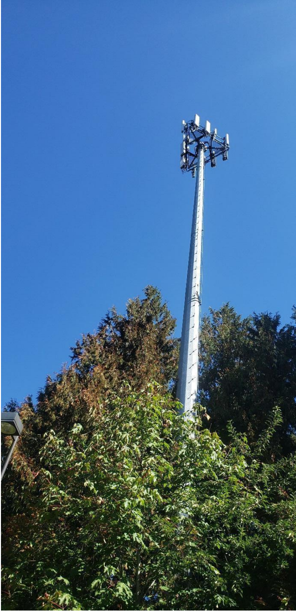
23. Cell tower on site of sampled fire station not detected by OpenCellID
